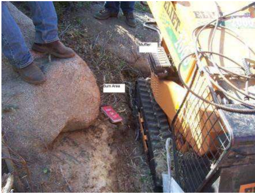
Figure 9. Area where small, spot fire was caused by chipped vegetation landing on the chipper exhaust at Tower 1044 (Photo from PAR incident Report).
