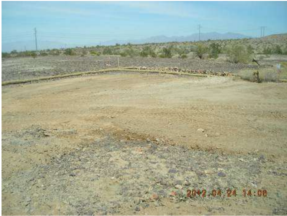
Figure 5. Spoils from foundation excavation placed on desert pavement at Tower 2524 (Photo Courtesy of Mark Augustyn).
