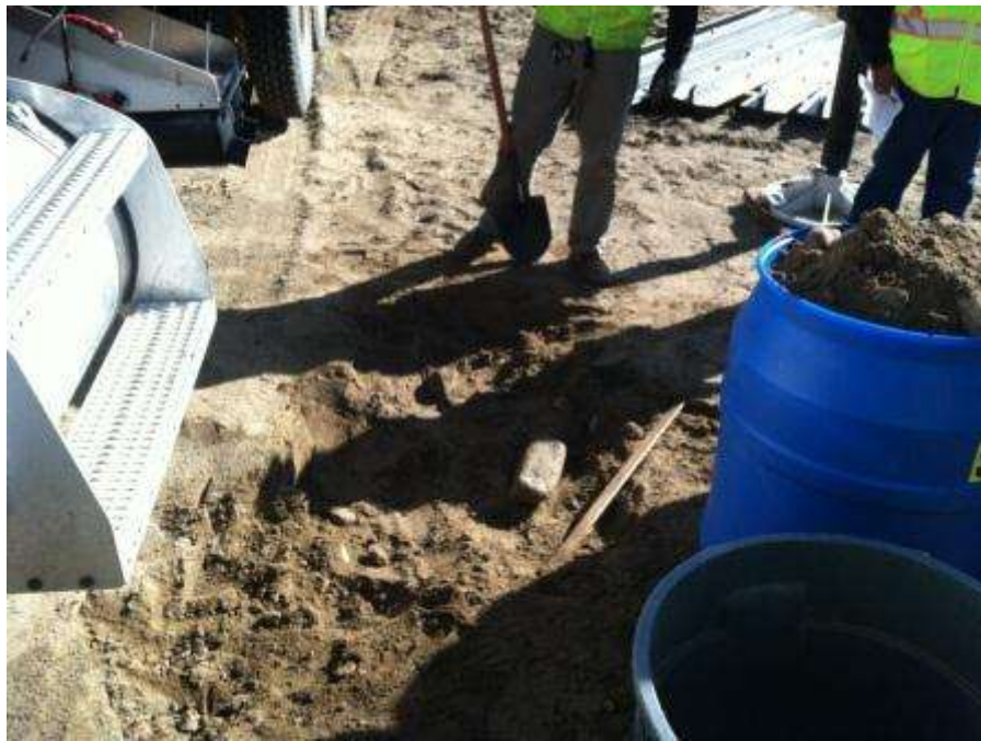
Figure 7. Diesel spill clean-up from resultant fuel spill as fuel was siphoned by thieves out of the crane parked onsite overnight (Photo Courtesy of Dean Ritter).
