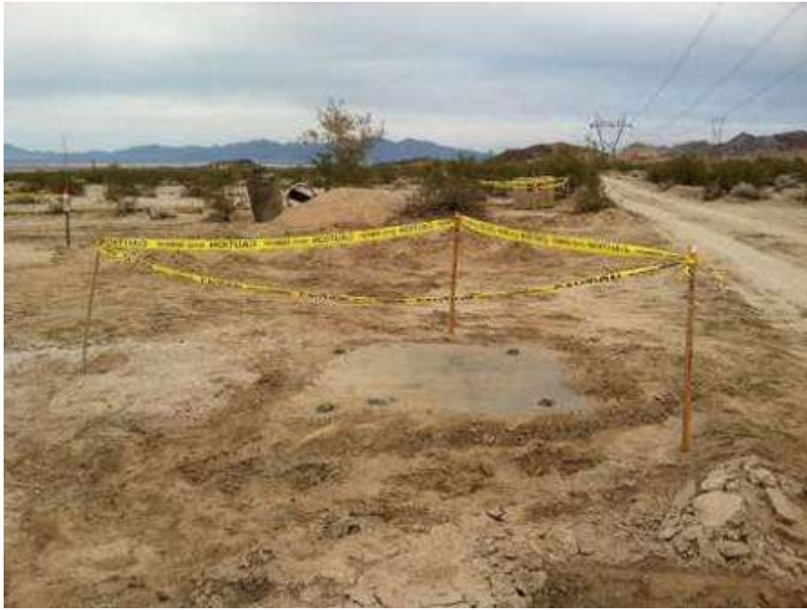
Figure 1. Covering of an open excavation at Tower 2523 was noted to be in compliance.
