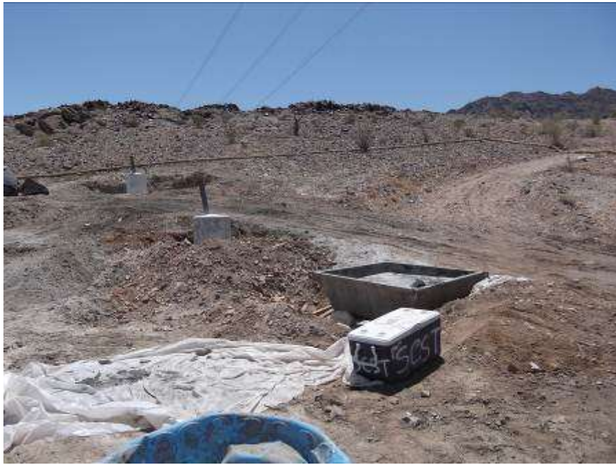
Figure 7. Concrete washout tub left uncovered at Tower 2518.
