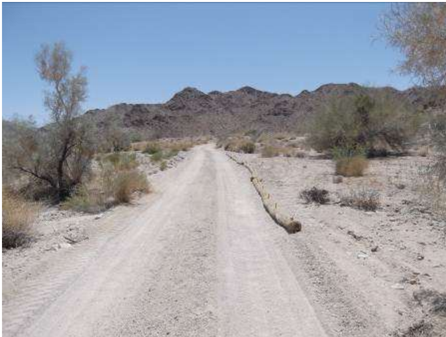
Figure 4. Straw wattles installed along access road near Tower 2425 to avoid off-road construction travel.
