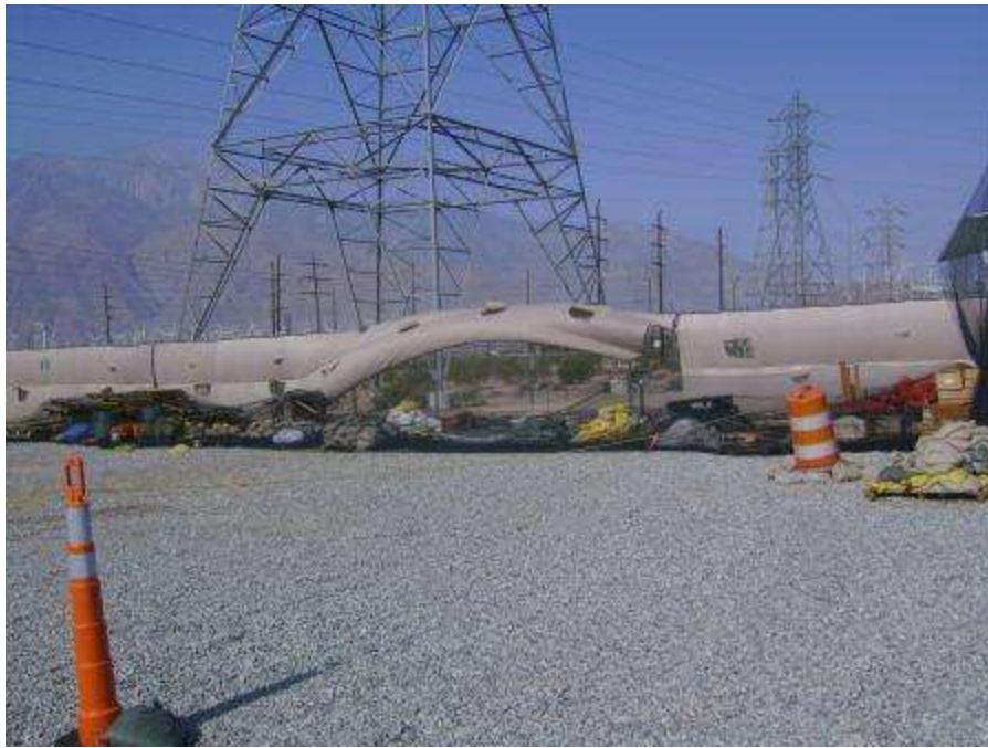
Figure 9. Construction yard screening at Devers Yard ripped away from fencing.
