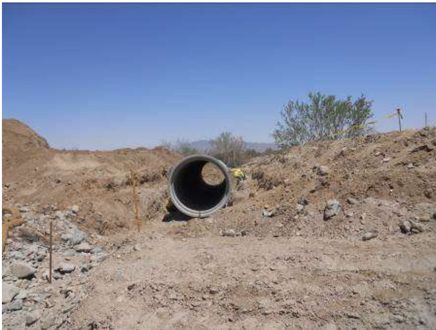
Figure 8. Installation of a culvert at a drainage crossing along Red Bluff access road.
