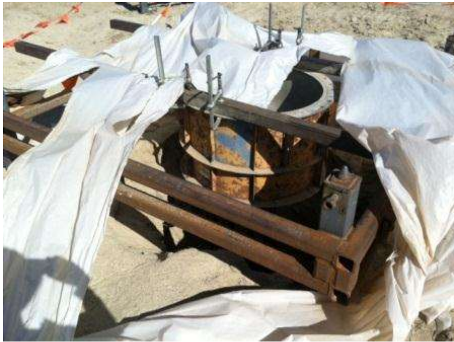
Figure 7. Inadequate covering of open hole excavation at Tower 2126.
