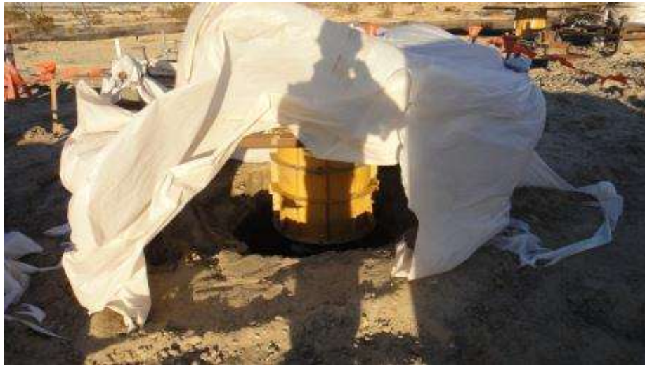
Figure 6. Inadequate covering of open hole excavation at Tower 2125.
