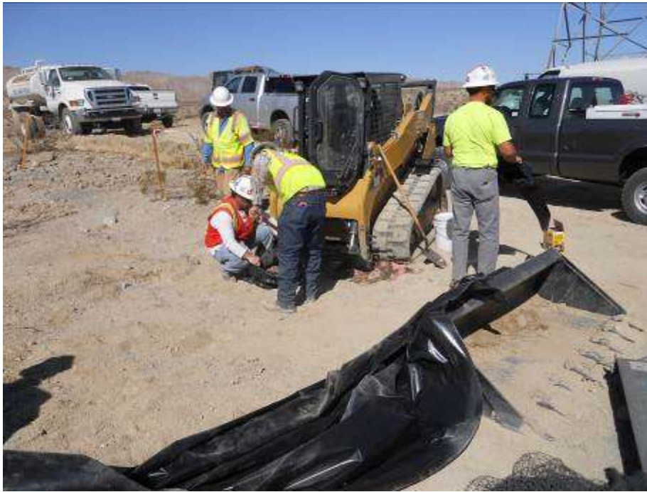
Figure 5. Crew working to remove contaminated soil due to hydraulic fluid spill at Tower 2266.
