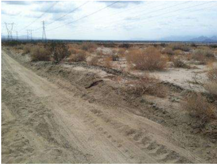
Figure 7. Impacts where a crane drove outside of the access road boundaries at Tower 2205.
