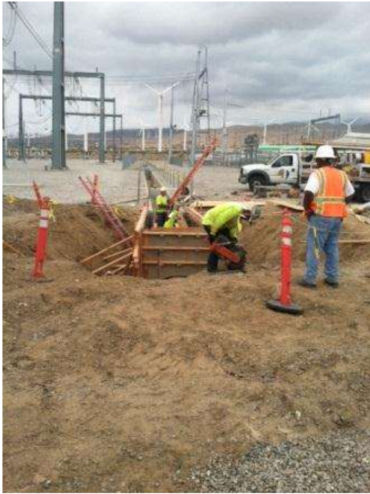
Figure 9. Trenching for a new waterline in the northern portion of the Devers Substation.
