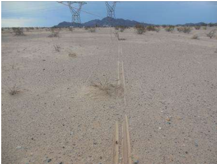
Figure 8. Area outside disturbance limits between Towers CR1-3W and CR1-4W where conductor wire accidentally touched the ground.
