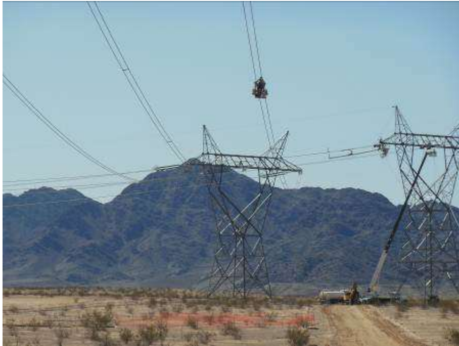
Figure 1. Adding spacers along the conductor during wire stringing activities at the CRS loop-in tower sites. The linemen ride in 'spacer carts' that travel along the conductor to install the spacers.
