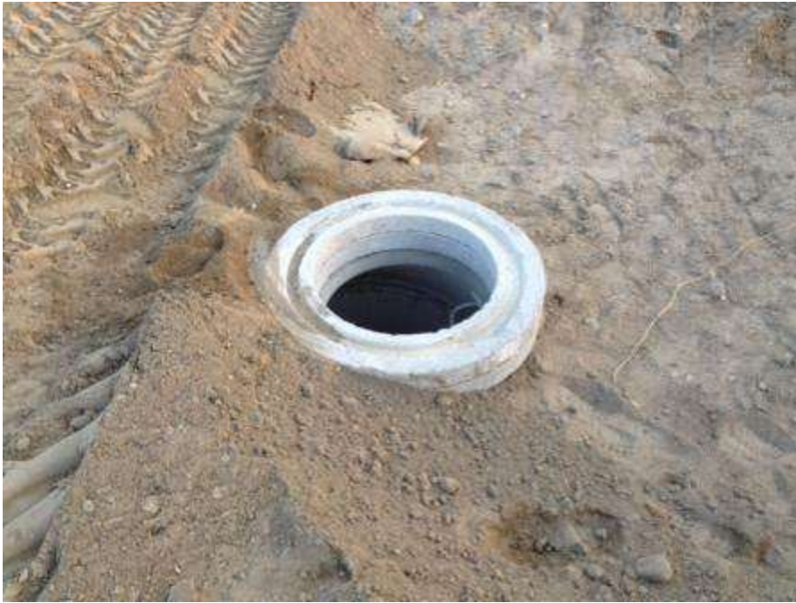
Figure 9. Manhole that was left uncovered overnight at the Devers Substation.
