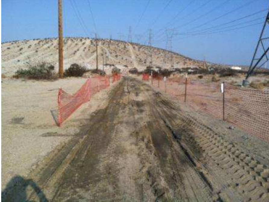
Figure 1. Construction fencing was placed at the boundaries of the access road to Tower 2110 to prevent off road impacts to Coachella Valley Fringe-toed Lizard habitat during access road grading and foundation excavation activities.
