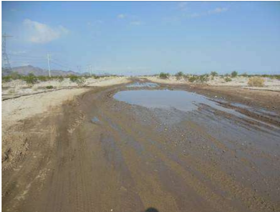
Figure 8. Heavy pooling along the Red Bluff access road due to recent rain.
