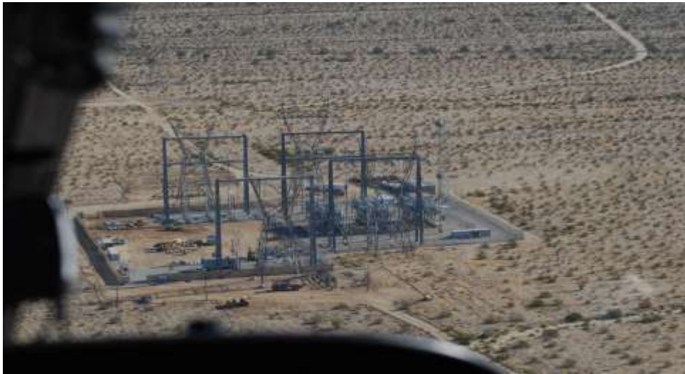
Figure 8. Overview photo of the Series Capacitor taken from the helicopter (photo provided by Kenny Construction).
