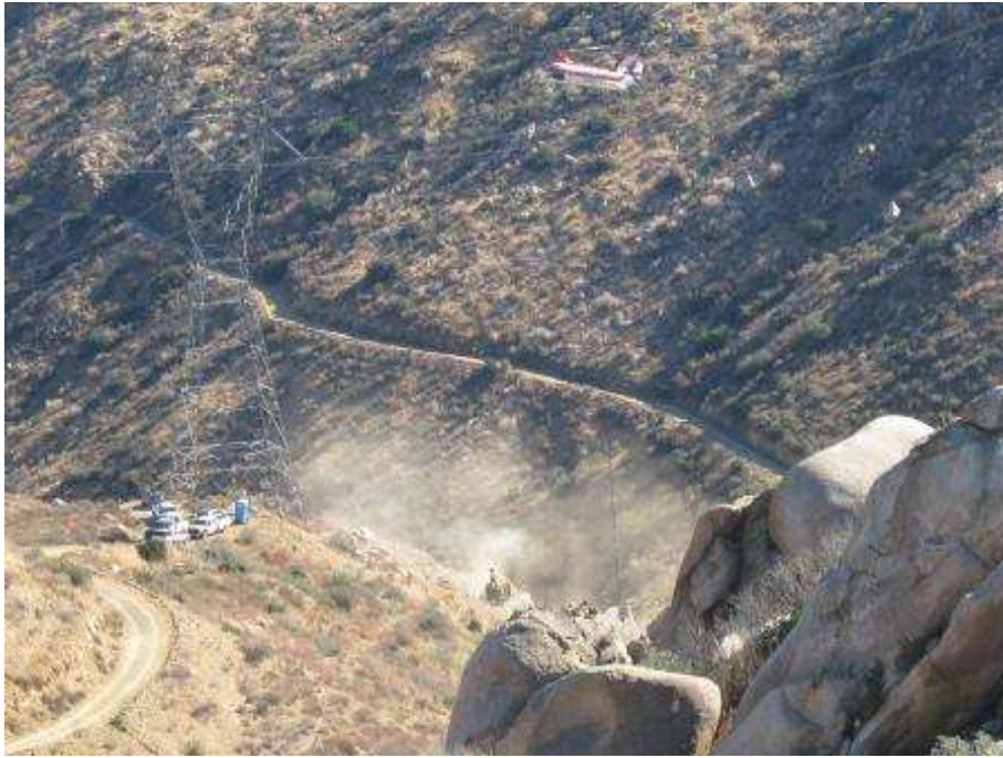
Figure 5. Inadequate dust control during helicopter operations at Tower 1070.
