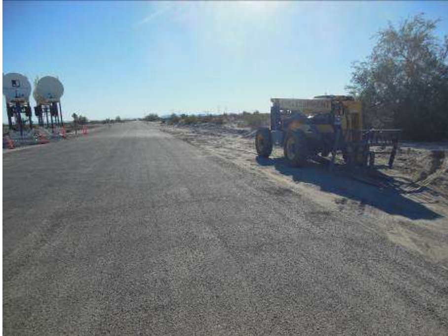
Figure 1. Forklift staged in unapproved area along Chuckwalla Road.
