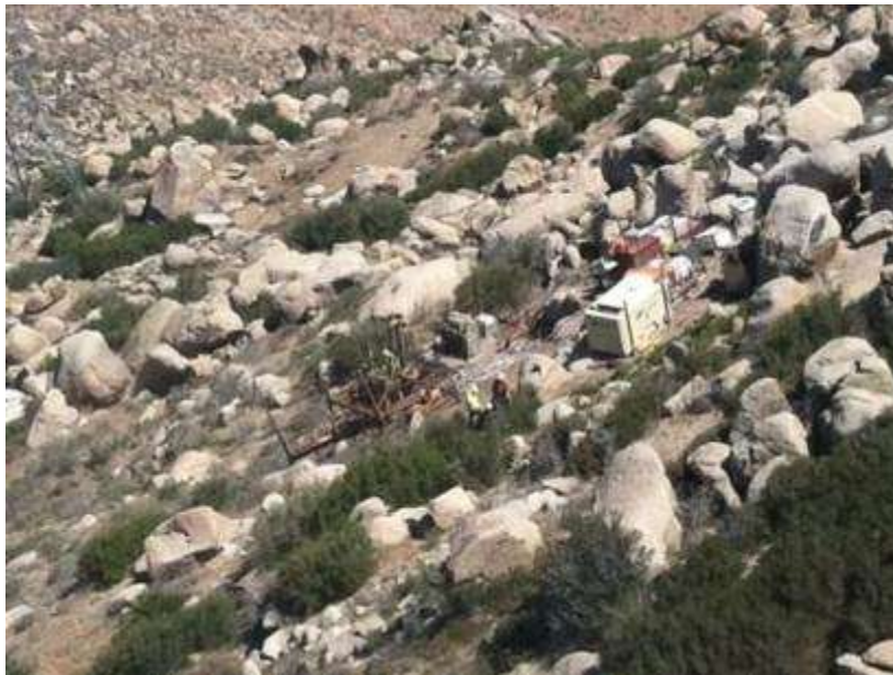
Figure 6. Micropile foundation drilling for the permanent platform at Tower 1046 (Photo taken from a helicopter).
