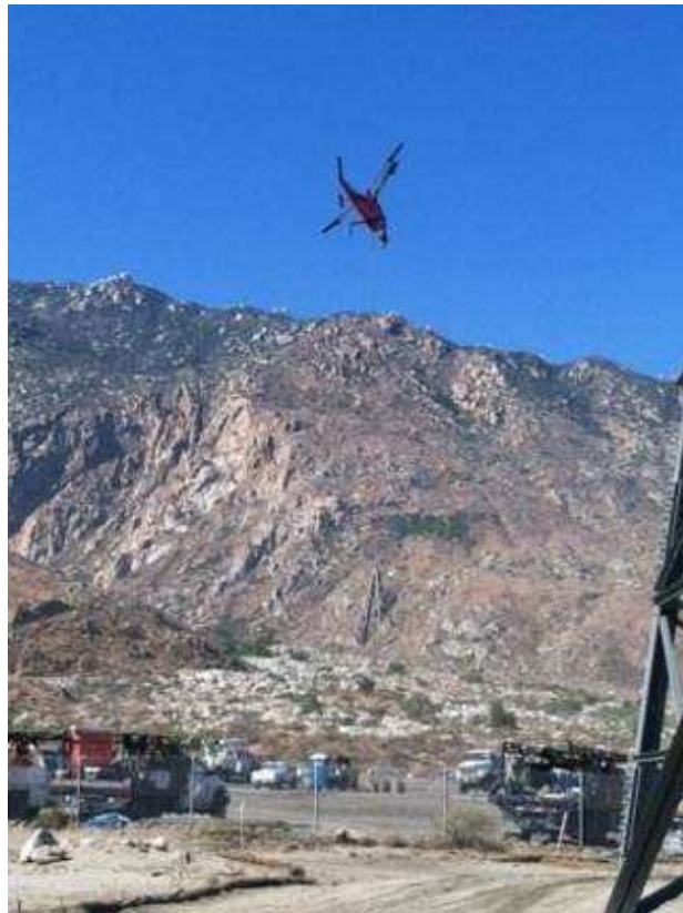
Figure 4. KMax helicopter lifting tower sections from HLZ H2 for tower assembly at a remote site
