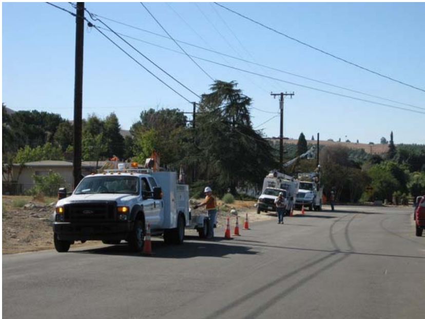
Figure 4: Installation of the framing arms and placement of pulling rope began at the intersection of Colton and Sapphire Streets in Mentone during the reporting period for the Mentone Substation to Zanja Substation portion of the Fiber Optic Cable installation. The photograph faces southward.
