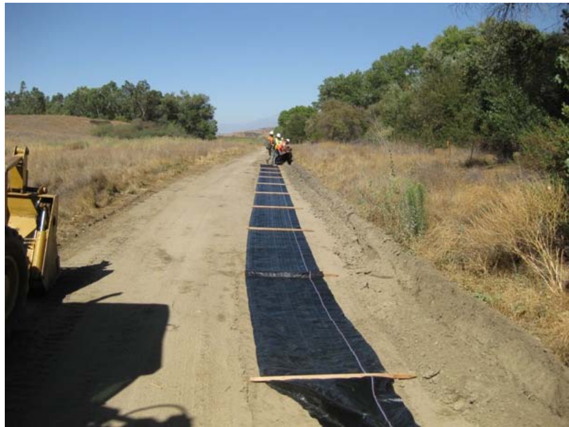
Figure 2: A silt fence installation along the north (San Timoteo Creek) side of the access road the entire distance from the entrance gate to the east end of the sub-station site. The photograph faces westward.
