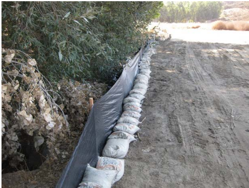
Figure 3: The culvert relocation site on the El Casco Substation access road was prepared with silt fence and sandbagging to protect San Timoteo Creek (to the left). The photograph faces eastward.
