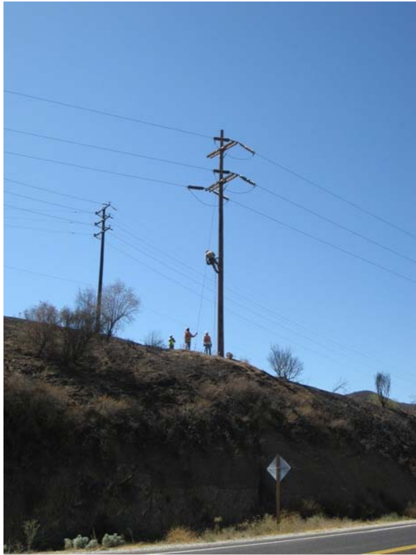
Figure 5: During the FOC installation work between Mentone and Zanja Substations, linemen climbed the poles in areas too remote for a bucket truck to approach. Biological Monitors directed the workers through sensitive habitats to the sites to avoid habitat disturbance. The photograph was taken from Highway 38, and faces southward.
