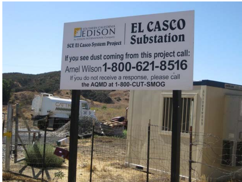
Figure 1: Construction activity at the El Casco Substation site began during the week of September 14, 2009. A temporary parking area was established just inside the entrance gate with a security guard building. The photograph was taken from San Timoteo Road, and faces southward.
