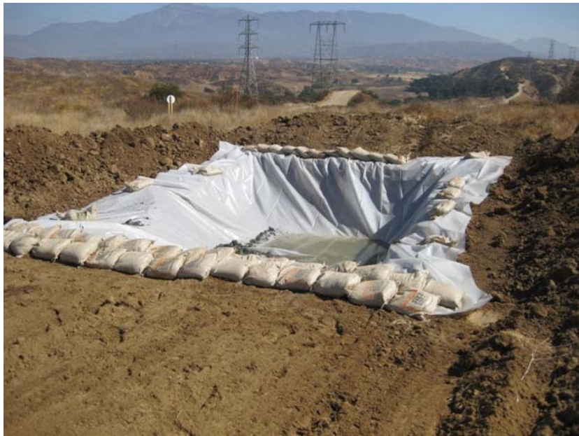
Figure 9: A concrete wash basin was built on the top of the hill at El Casco Substation site in order that concrete trucks supplying the terrace work can be cleaned before the residue concrete dries inside the trucks. The photograph faces eastward.
