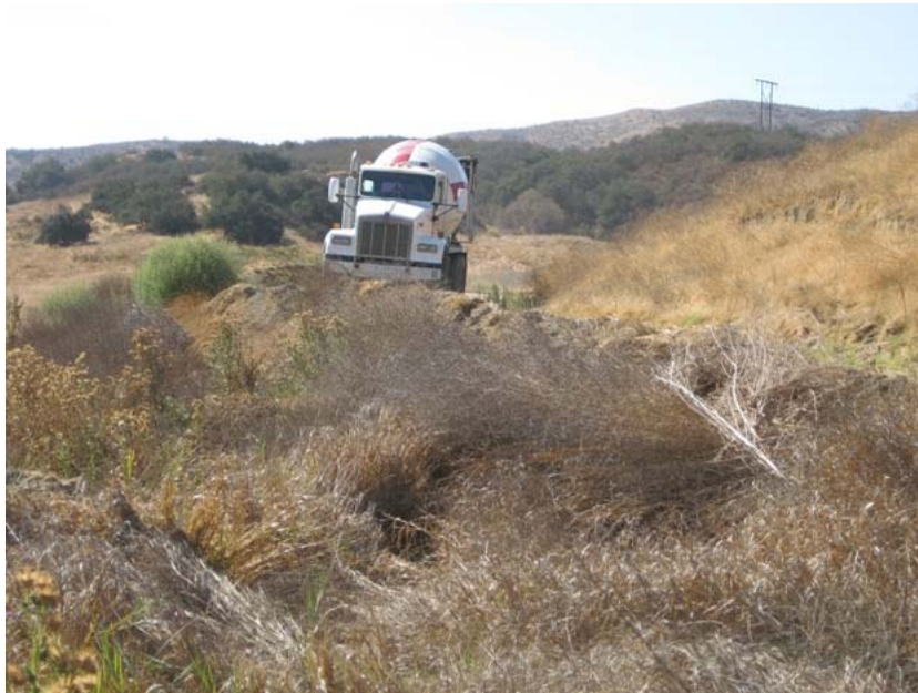
Figure 10: Access roads south of the El Casco Substation site are being used to reach the top of the hill within the Substation site with vehicles, equipment, concrete trucks, and water trucks. These are pre-existing roads. There will be no disturbance of natural habitat off the roads. The roads are being watered regularly for dust control. The photograph faces eastward.
