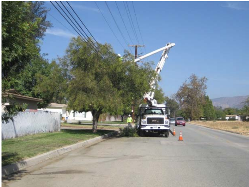
Figure 7: During the subject week, tree-trimming for FOC installation occurred on Bryant Street in Yucaipa. A biological monitor (to the left of the truck) accompanied the crew at all times. The photograph faces southward.
