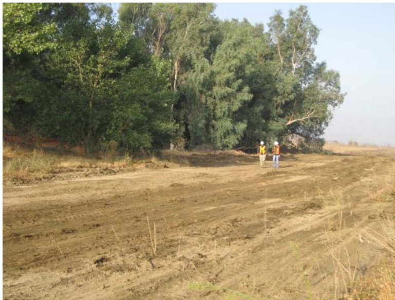
Figure 3: The grading of the new access road to El Casco Substation began during the subject week. California walnut and cottonwood trees at the edge of the grove in the background were avoided. The grading activity was accompanied by biological and cultural resource monitors at all times. The photograph faces westward.
