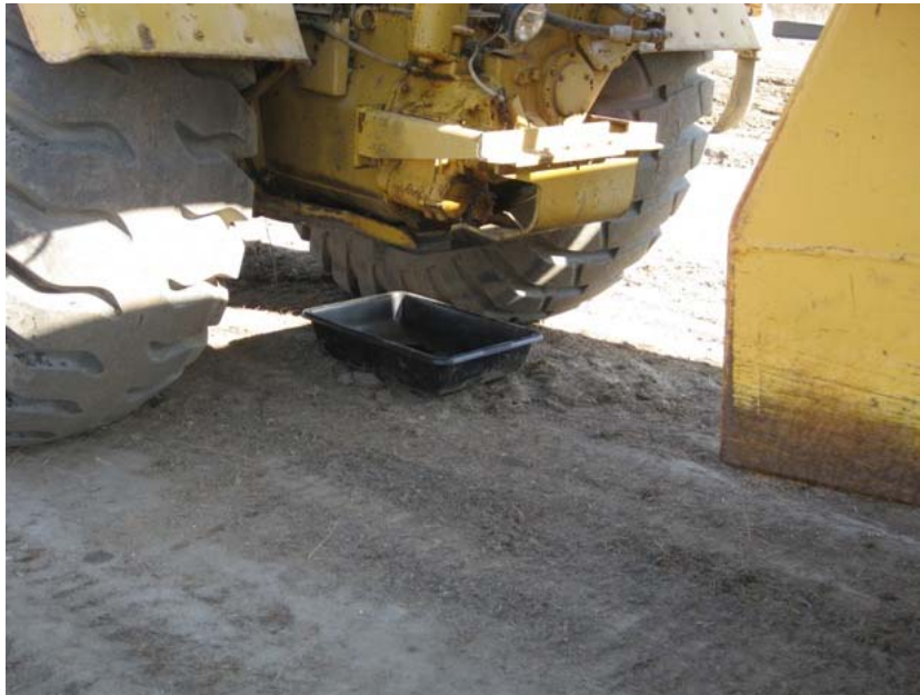
Figure 8: Equipment and vehicles were checked regularly for fluid leaks. This paddle-wheel excavator at the El Casco Substation staging area has been fitted with a drip pan until it is repaired.
