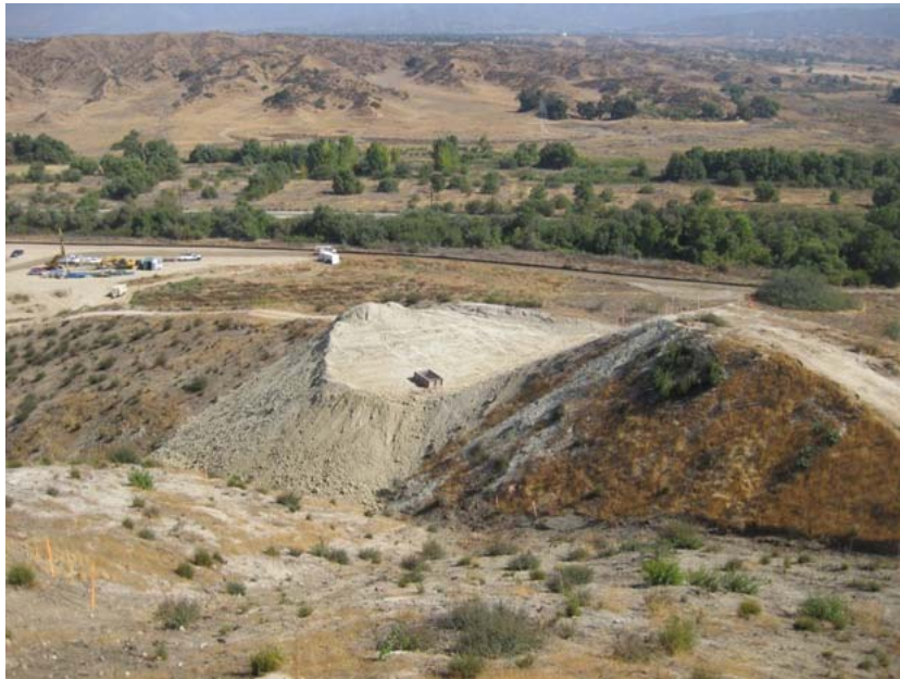
Figure 4: Terracing of the hillside began on Wednesday of the prior week. Fourteen terraces will be constructed in stair step fashion on two prominent ridges of the hillside. There will be four terraces on the ridge in view, and ten on another ridge to the left of the photograph. The staging area is in the distance on the left. The photograph faces northward.
