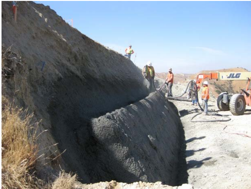
Figure 5: The face of each terrace will be fitted with a tie-back structure that will provide an anchor for an approximately 120 foot long cable placed in an oblique bore dug into the hill.
