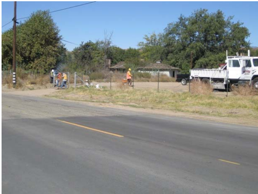
Figure 4: Preparation of the site for the second water pipeline/tower system began adjacent to San Timoteo Canyon Road. A gate and fencing was being placed in front of the site of the water tower during the subject week. The photograph faces northwestward.
