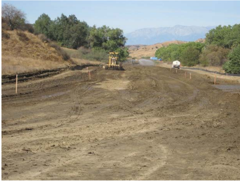
Figure 1: Grading work on the new access road to the El Casco Substation site continued during the subject week. Five cottonwood trees behind the grader will be removed to allow for construction. The photograph faces westward.
