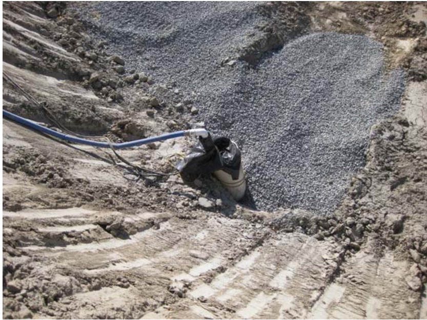
Figure 6: The inner well of the dewatering operation at the El Casco Substation site was filled with gravel to prevent entrapment of animals.
