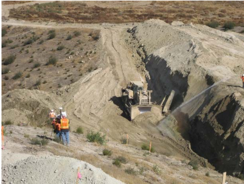
Figure 2: On the hillside at the El Casco Substation site, the contractor began constructing the second set of terraces. The photograph faces northwestward.
