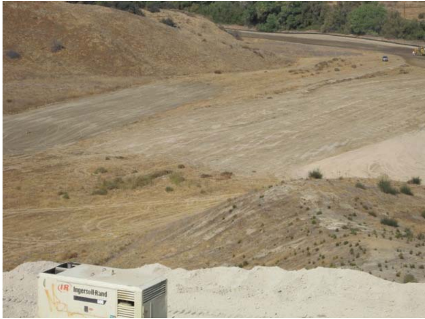
Figure 5: A flat area on the southwestern side of the substation site was cleared of vegetation during the subject week in preparation for installation of SCE project field trailers. The photograph faces northwestward.
