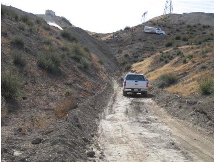
Figure 3: On the hillside at the El Casco Substation site, the gully between the ridges is being filled in as the operation proceeds. The photograph faces southeastward.
