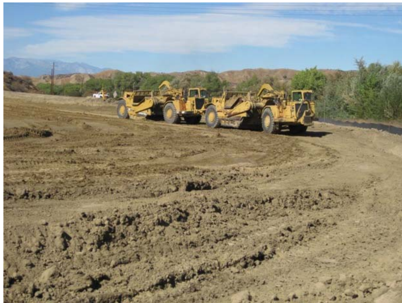
Figure 2: The material for the heightened road is being hauled in from the over-excavation area of the substation site. This area is being over-excavated to allow the placement of a more firm base for the substation. The photograph faces northwestward.
