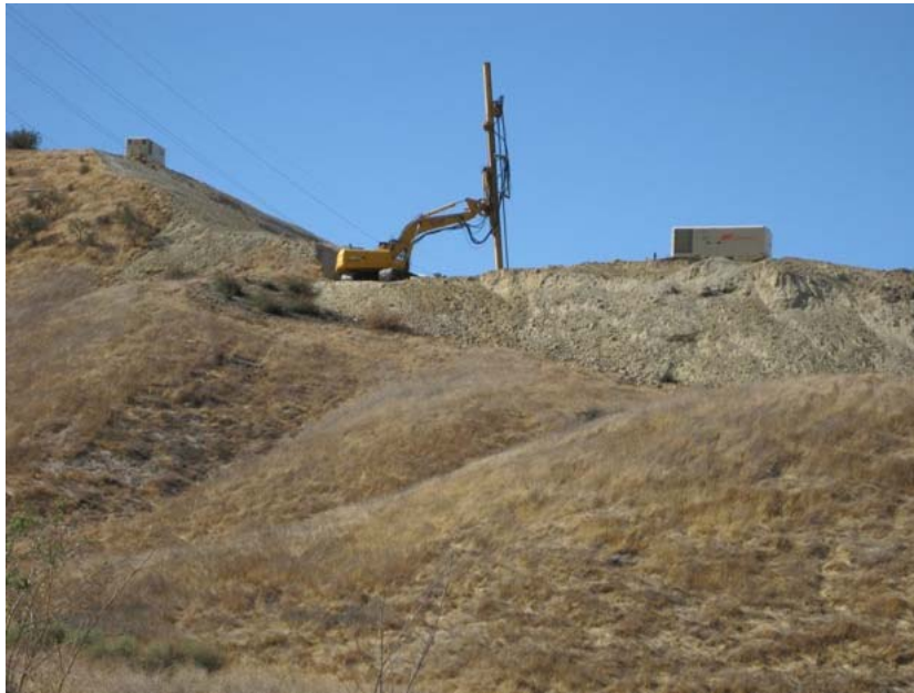
Figure 3: During the subject week, the second terrace on each of the two ridges was excavated. Construction of the tie-in wailers and boring of the anchor holes at the second terraces began. An anchor hole is being bored at terrace N. The tie-ins at Terrace M, above it, have been backfilled. The second, higher ridge is out of sight. Its terraces begin with A at the top. Terrace B is under construction presently. The photograph faces southeastward.
