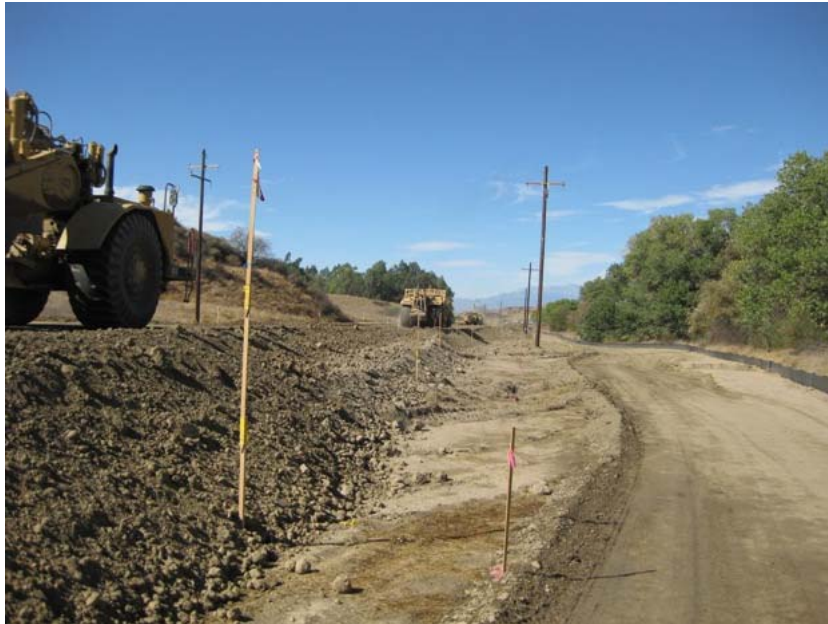
Figure 1: During the subject week, grading of the new access road continued. The new access is being raised several feet above the original ground level, and the level of the pre-existing access road on the right. The photograph faces westward.
