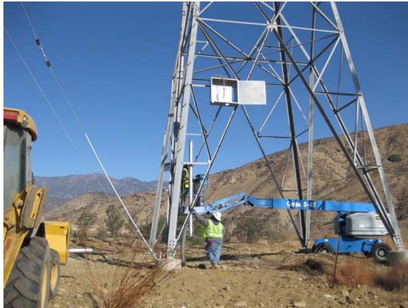
Figure 3: Recently installed underground conduit was connected to Tower M12T2 via a steel riser and a 3x3 box at the north end of the Banning to Tower M17T2 FOC segment on Bluff Road. The photograph faces northward.
