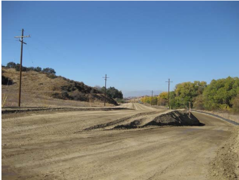
Figure 1: The utility line installation for the construction site field office trailers at the El Casco Substation site was completed by SCE FOC crews during the second week of the subject period. The new access road is on the left; the pre-existing road is on the right. The photograph faces westward.
