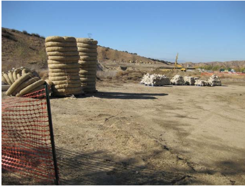
Figure 5: Several significant storm events are predicted beginning Monday of the following week. At El Casco Substation site several measures have been implemented or are ready to be implemented including the placement of straw wattling and sand bags. The photograph was taken at the substation site and faces southwestward.
