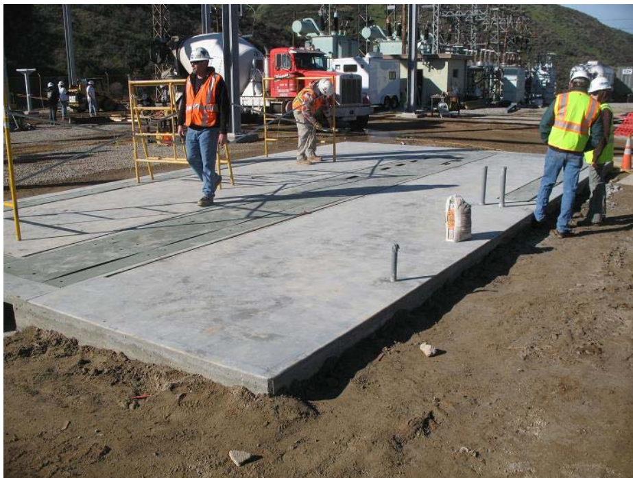
Figure 6: View of completed MEER building foundation at the Zanja Substation. The photograph faces southwestward
