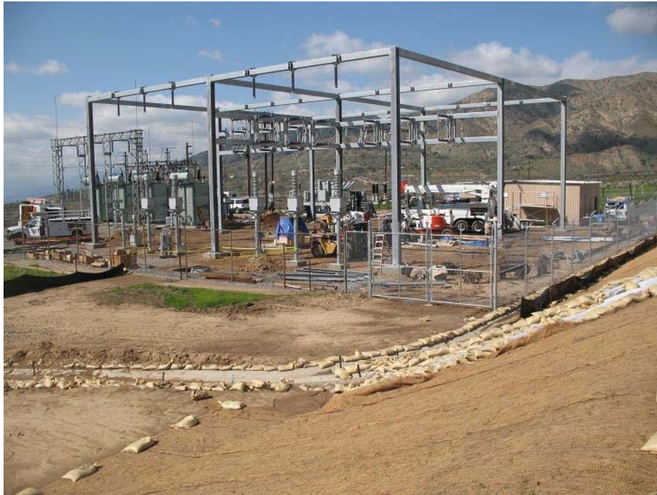
Figure 7: View of the completed rack and MEER building at the Zanja Substation. The photograph faces northwestward.
