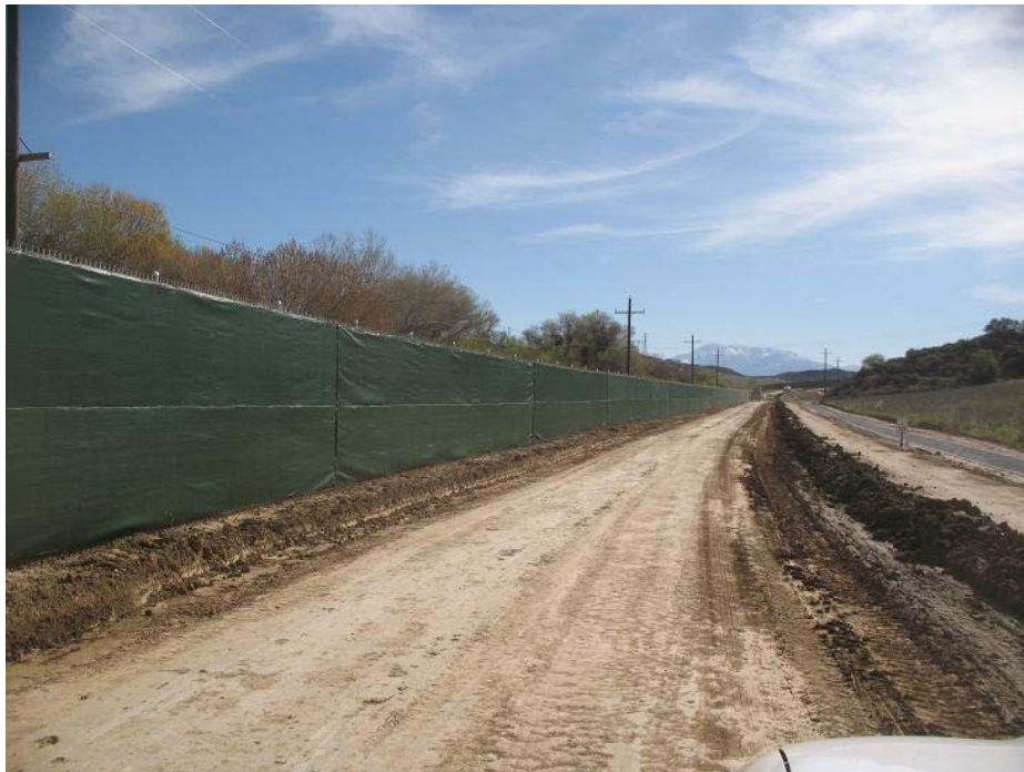
Figure 4: View of completed chain link fencing along the access road. The photograph faces eastward towards the substation site.
