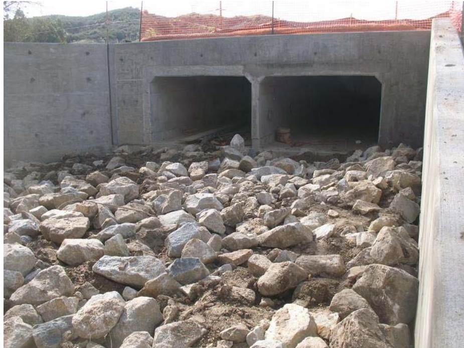
Figure 2: View of completed box culvert outlet near El Casco Substation entrance. The photograph faces southward.
