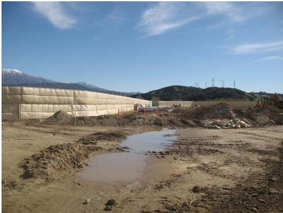
Figure 5: View of the nearly completed chain link fencing around the El Casco Substation pad. The photograph faces northeastward.
