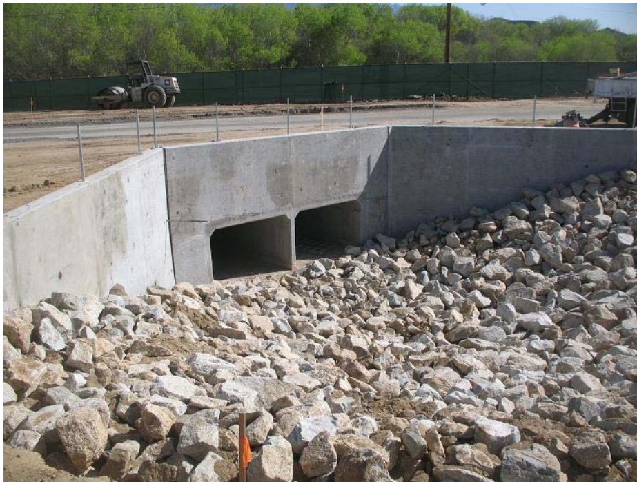
Figure 3: View of completed box culvert inlet near El Casco Substation entrance. The photograph faces northward.
