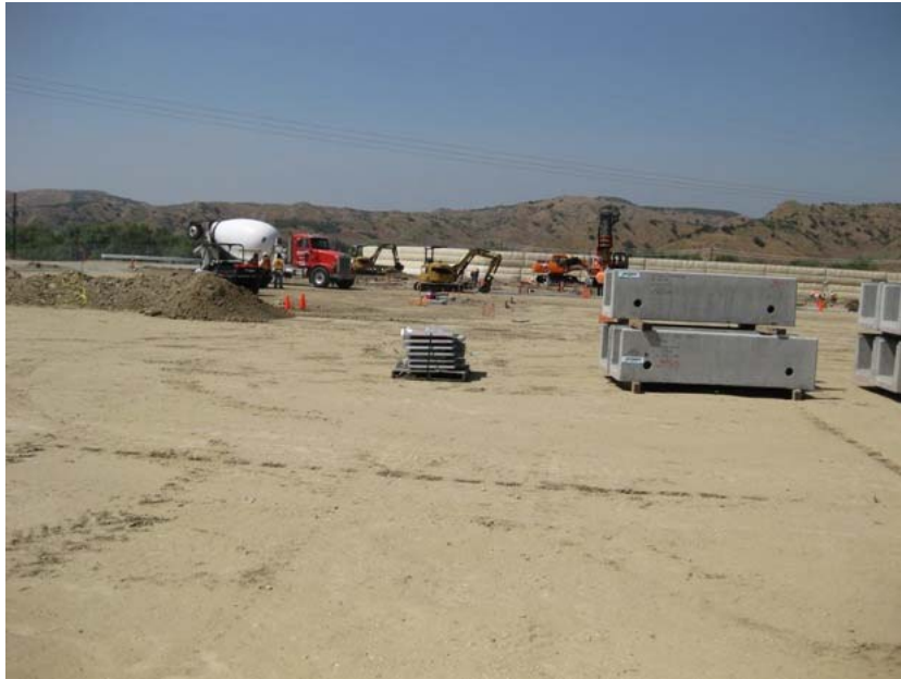
Figure 1: Work at the El Casco Substation site continued with trenching for ground wire placement, preparing trenches for conduit placement, and constructing foundations for structures. The photograph faces northeastward.
