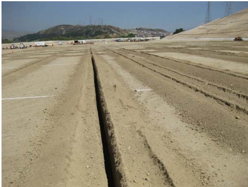
Figure 4: Temporary trenches were being dug on the pad at the El Casco Substation site for the copper grounding wire grid. These trenches have the potential to trap animals. NRC Biological Monitors inspected the trenches each morning, using flashlights when necessary, for trapped individuals. The photograph faces northeastward.
