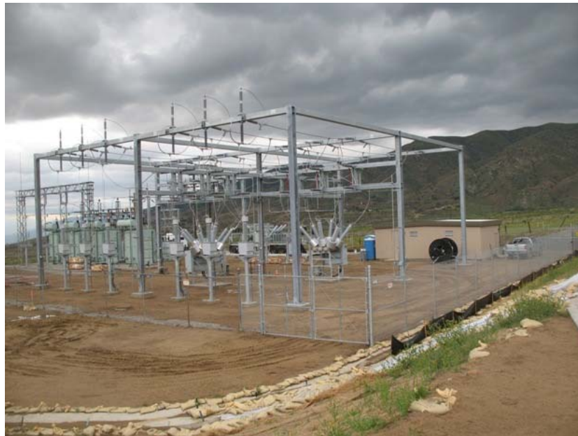
Figure 2: Construction activity at the Zanja Substation has been mostly completed. Work continued within the substation on the installation of the new electrical components. The photograph faces northwestward.
