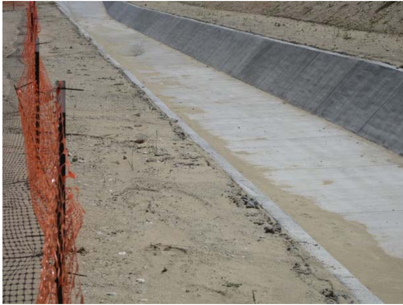
Figure 5: Permanent V-ditches that have been constructed on the periphery of the El Casco Substation site may have the potential for entrapment. The issue is being investigated further by SCE. The photograph was taken between the office trailers and the substation pad, and faces southward.
