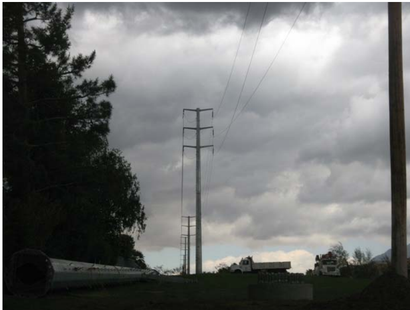
Figure 3: Installation of Segment 3 of the 115 kV sub-transmission line within the Sun Lakes development in Banning has been completed.
