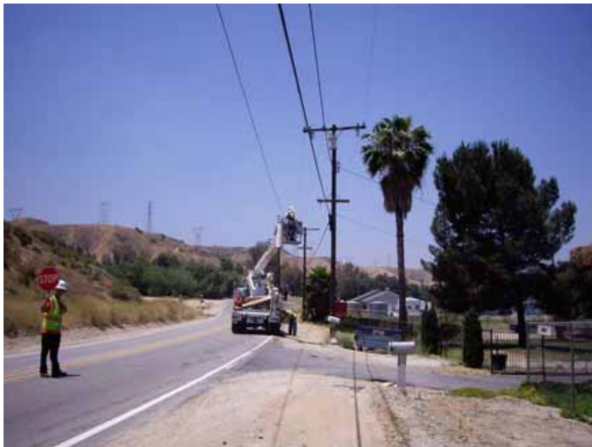
Figure 3: Fiber optic cable work along San Timoteo Canyon Road. This photograph is taken facing west.
