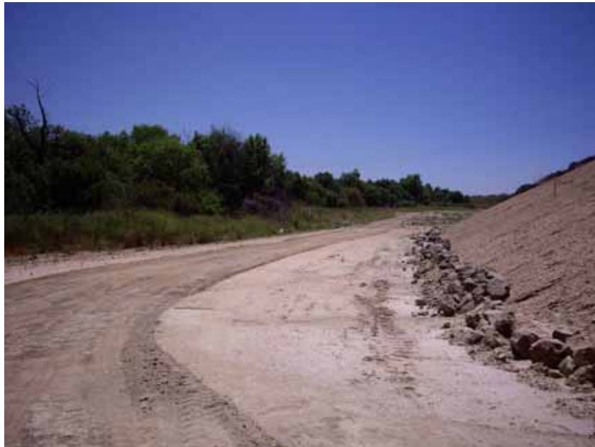
Figure 5: Grading activity along access road. Known least Bell's vireo territory is on the left. This photograph is taken facing southeast.
