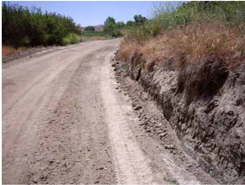
Figure 4: Grading activity along access road near El Casco Substation. San Timoteo Creek is to the left of the access road. This photograph is taken facing southeast.
