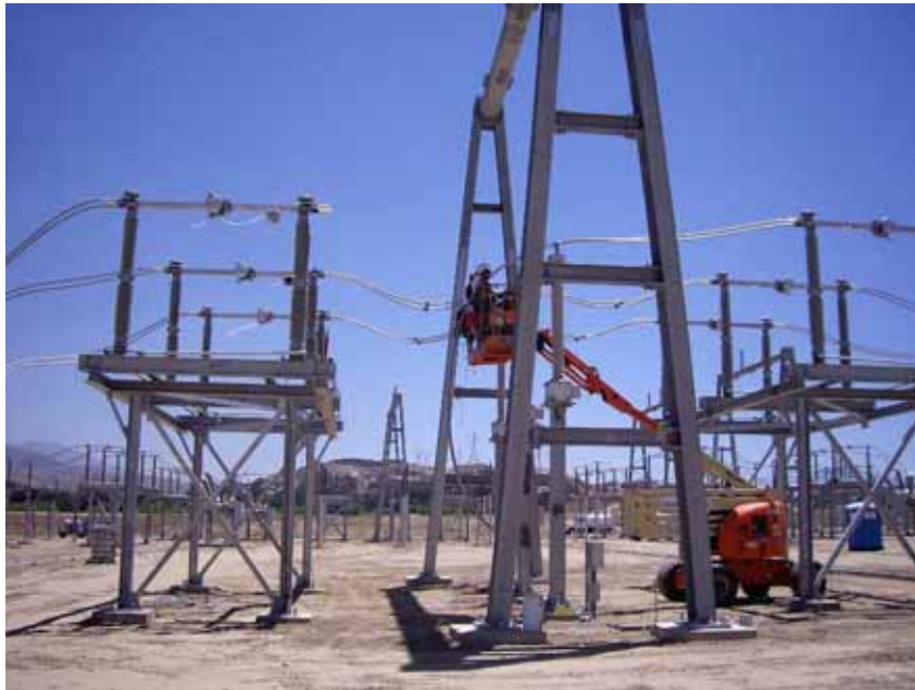
Figure 2: At the El Casco Substation, crews continued to work on the 220 kV switchrack structures. This photograph is taken facing east.
