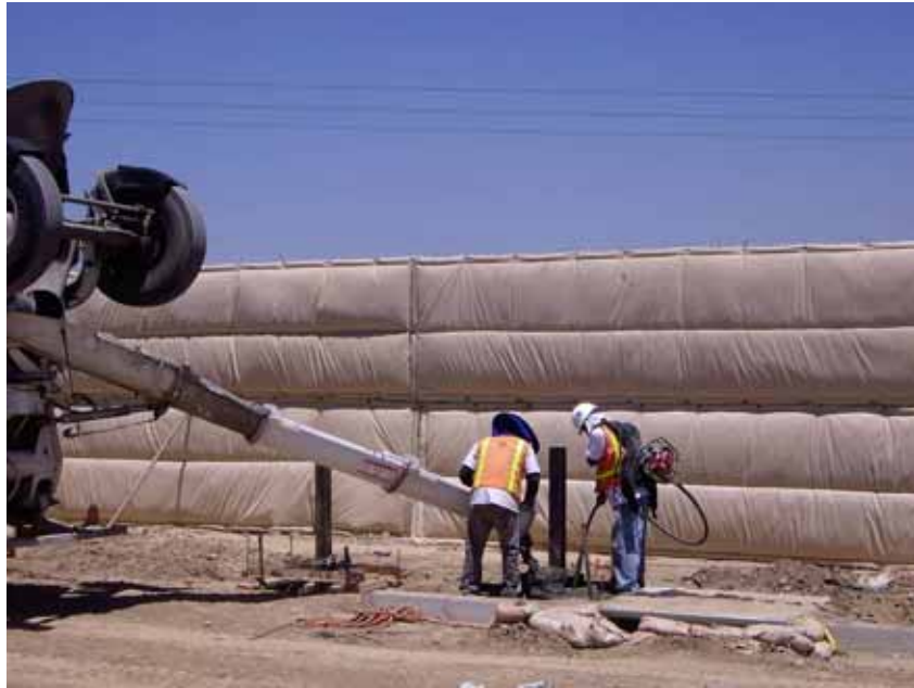
Figure 1: At the El Casco Substation site, crews poured concrete into a trench for the grounding grid system. This photograph was taken facing north.
