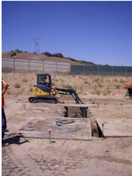
Figure 4: Work on the foundations of three towers on the lower pad. The photograph is taken facing south.
