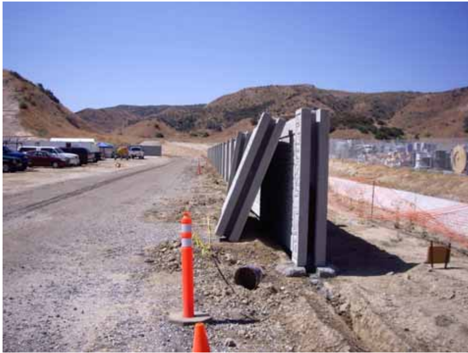
Figure 3: At the El Casco Substation site, work continued on the perimeter wall. The photograph is taken facing south.
