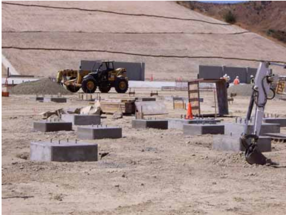
Figure 1: At the El Casco Substation site, crews worked on foundations for the AA banks for the 220 kV switchcracks. The photograph is taken facing south.
