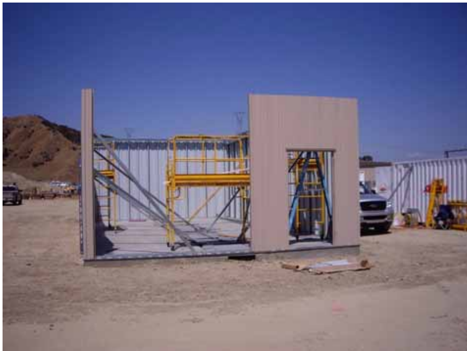
Figure 2: At the El Casco Substation site, work advanced on the 115 kV MEER building. The photograph is taken facing east.
