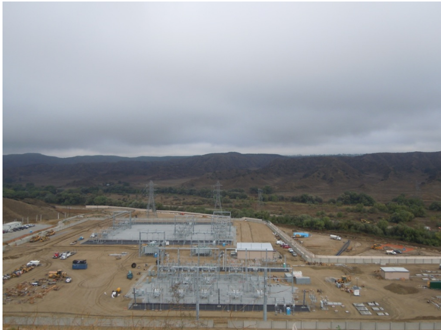
Figure 4: At the El Casco Substation site, a view of the substation from atop the slope at the southern end of the site. The three new 220 kV towers are visible in the background as well as the HDD bore exit side.
