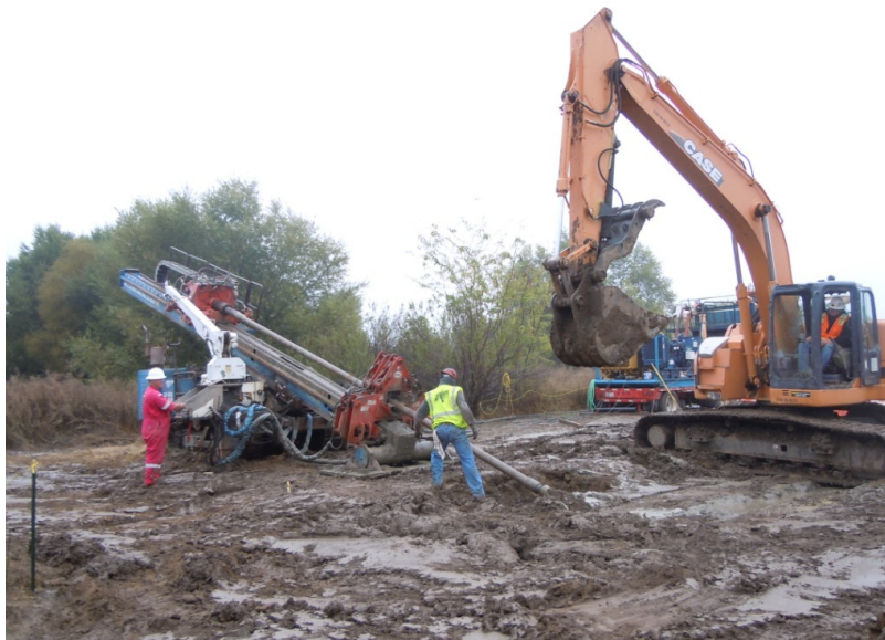
Figure 2: Along San Timoteo Canyon Road, the drilling rig at the bore entry side.
