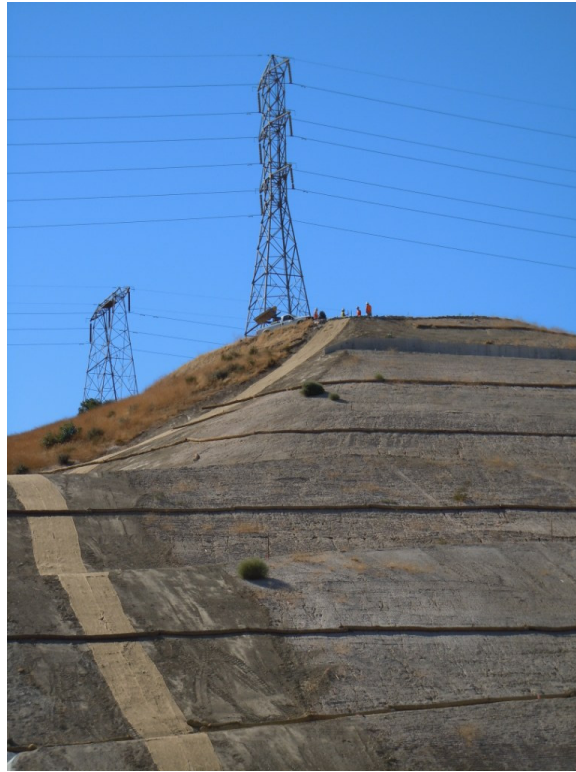
Figure 1: At the El Casco Substation site, crews worked on installing telephone conduit in the southern slope of the site. Netting was put in place to prevent erosion.
