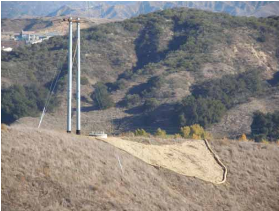
Figure 3: At the El Casco Substation subtrans site, newly installed fiber rolls at a foundation site.
