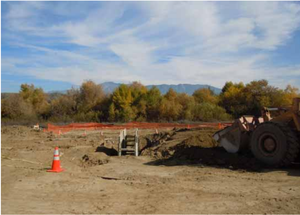
Figure 1: At the El Casco Substation site, HDD crews work on pulling conduit through one of three bore casings.
