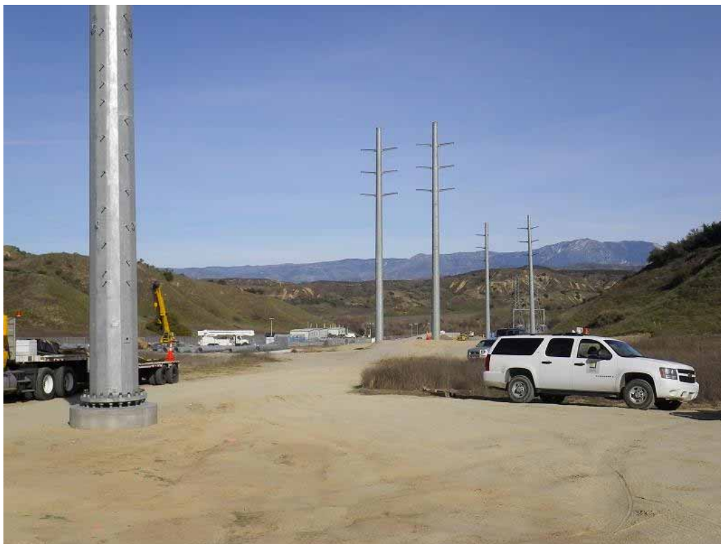
Figure 4: View of recently installed tubular steel poles just south of the El Casco Substation. The photograph faces north.
