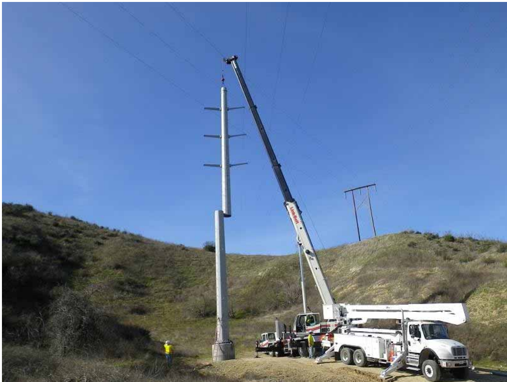
Figure 3: View of tubular steel poles being installed just south of the El Casco Substation. The photograph faces southwest.
