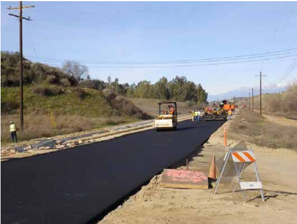
Figure 2: View of paving activities at the El Casco Substation access road. The photograph faces west.
