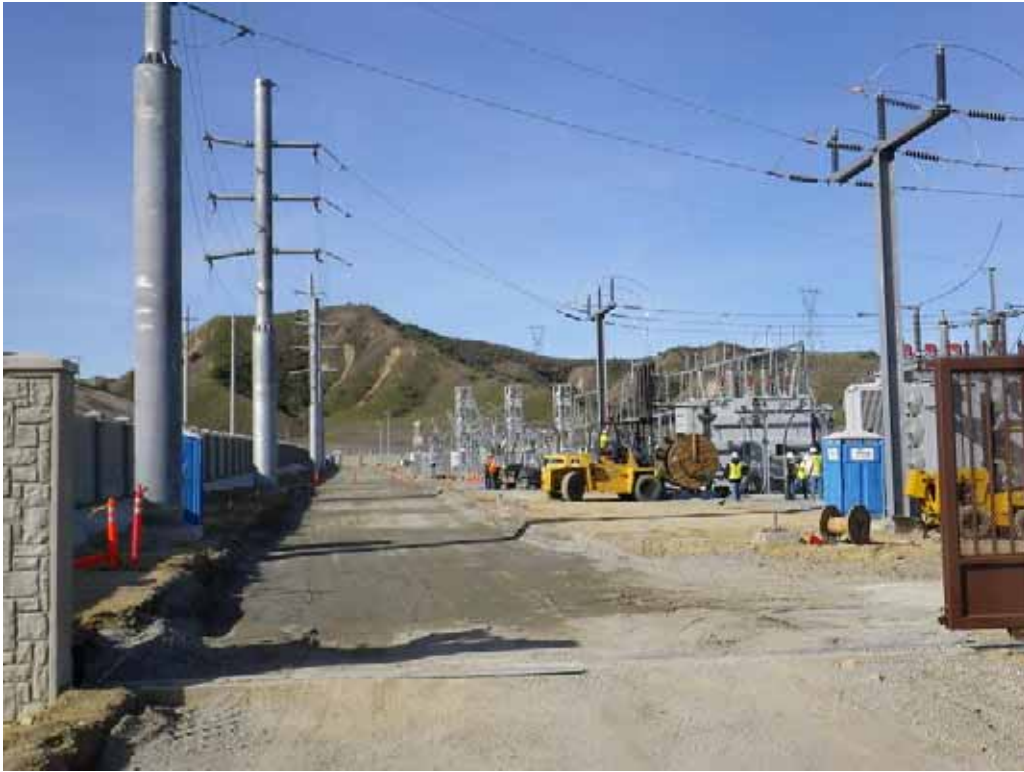
Figure 1: View of activities with the El Casco Substation. The photograph faces west.
