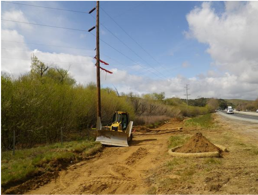
Figure 2: View of work in the vicinity of pole 207, the trimmed riparian vegetation is immediately to the left of the existing pole. The photograph faces west.
