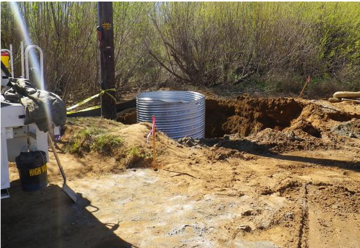
Figure 2: View showing the foundation of pole 207 on Segment 7 after the foundation had been removed and a second installation attempt was made. The photograph faces south.
