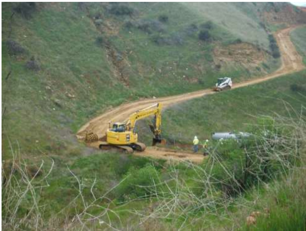
Photo 4 – Access road recontouring between Construction Areas 4X06 and 4X07, Segment 4 (March 24, 2020) (Photo courtesy of SCE).
