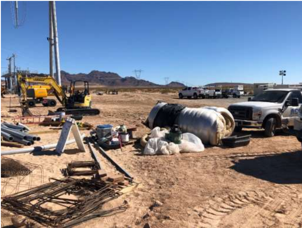
Photo 3: Reception of MEER equipment/hardware at Ludlow Series Capacitor (February 8, 2022).
