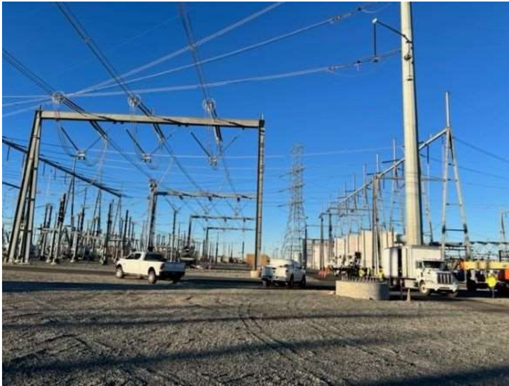
Photo 3: Wire stringing at SC4, Lugo Substation (November 10, 2022; photo by Matteo Daniel, Rincon).
