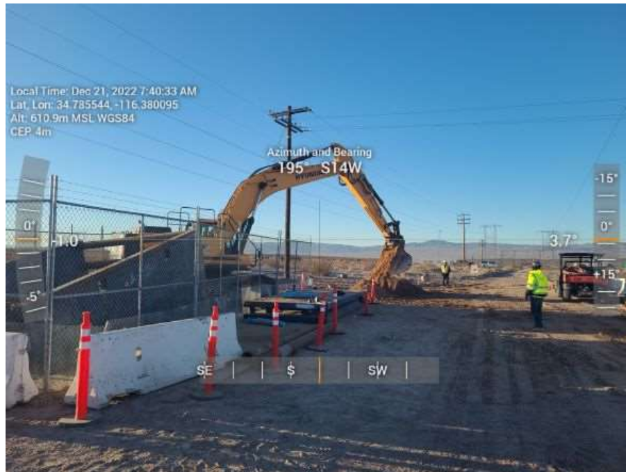
Photo 3: Excavating bore pits for railroad crossing outside SC5 (December 21, 2022; photo by Nick Barth, EPC).
