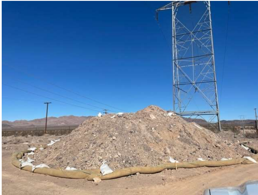
Photo 3: Refuse material from trenching and foundation pouring outside SC5 (January 25, 2023).
