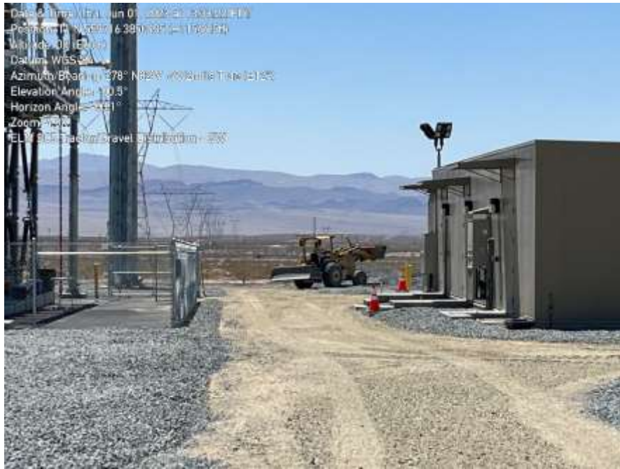
Photo 1: Backhoe activity (gravel distribution) at SC5, bringing site to final grade on June 1st.
