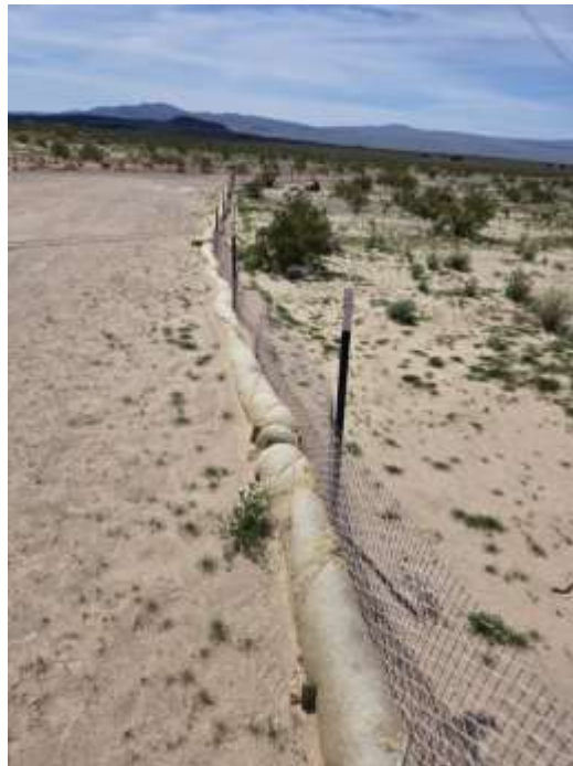
Photo 4: Newly-installed (February) perimeter BMP replacements at the perimeter of SC5. Some minor animal damage evident. Photo courtesy of site QSP, SWPPP inspection conducted on March 27th, 2024.
