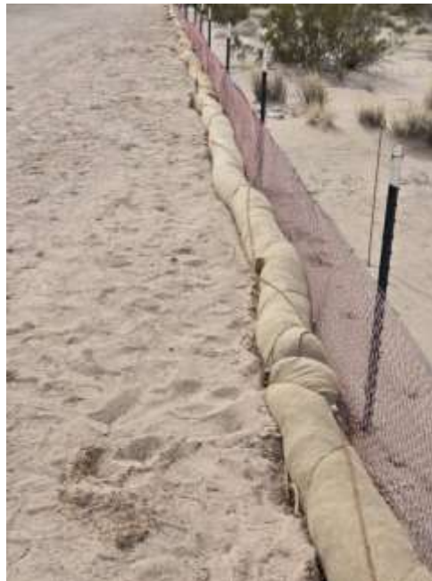
Photo 2: New perimeter wattle BMP replacements installed at perimeter of SC5. Photo courtesy of site QSP, SWPPP inspection conducted on February 14 th , 2024.
