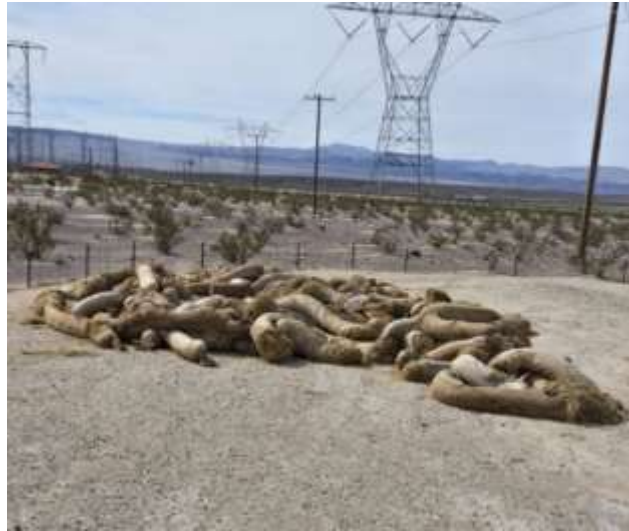
Photo 1: Stockpile of damaged wattles that have been removed from both perimeter fence lines and stockpiles on-site at SC2. Removal from site is pending. Photo courtesy of site QSP, SWPPP inspection conducted on February 14 th , 2024.
