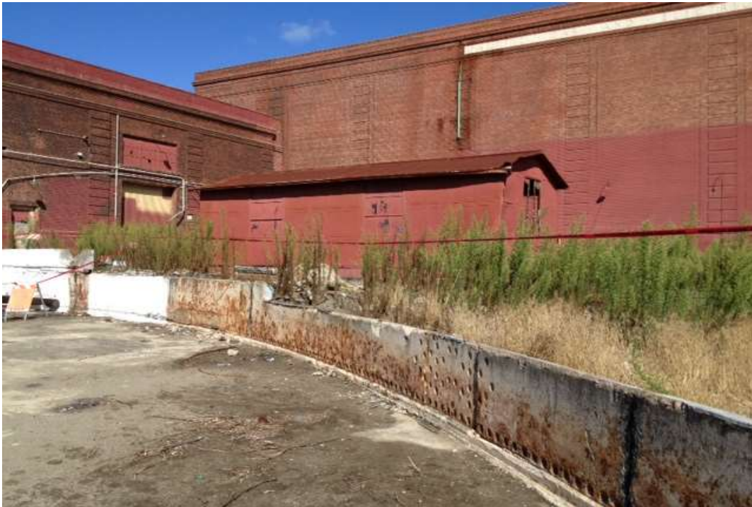
Figure 1 – Shed (Structure 1) and wall to be treated for asbestos at Potrero Switchyard. View northeast, September 25, 2014.
