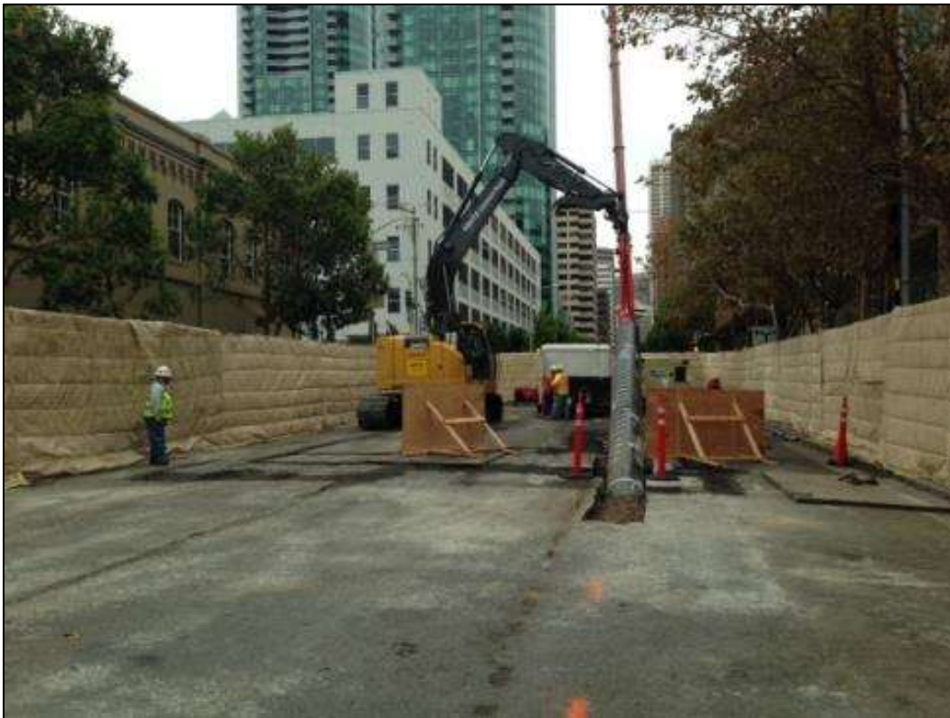
Figure 2 – Sound wall surrounding Spear Street HDD work area. View west, September 20, 2014 (photo courtesy of PG&E).
