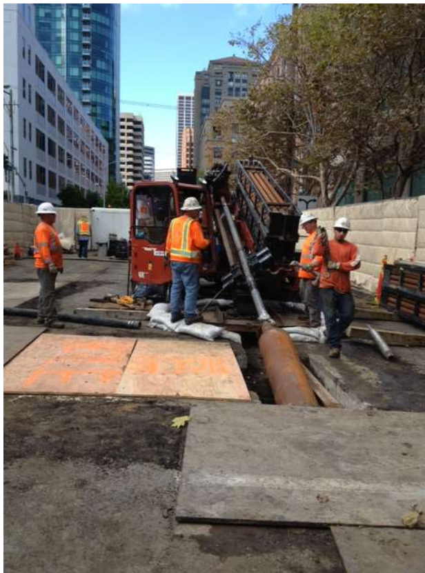
Figure 3 – HDD rig staged on Spear Street with supporting equipment and sound wall surrounding work area. View west, September 25, 2014.
