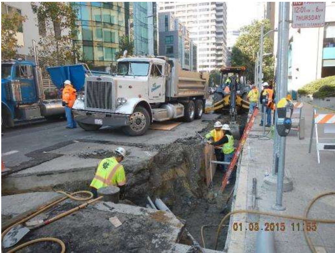
Figure 3 – Excavating for utility relocation on Spear Street. View west, January 3, 2015. Photo courtesy of PG&E.
