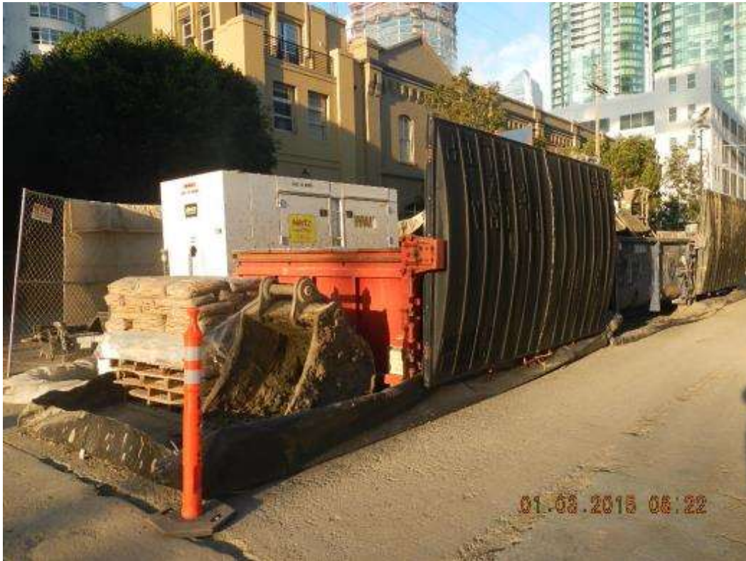
Figure 1 – HDD North secondary containment for bentonite. View southwest, January 3, 2015. Photo courtesy of PG&E.
