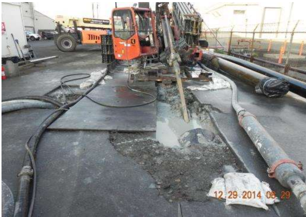
Figure 2 – HDD Company drilling at Bore 3 at HDD South. View west, December 29, 2014. Photo courtesy of PG&E.
