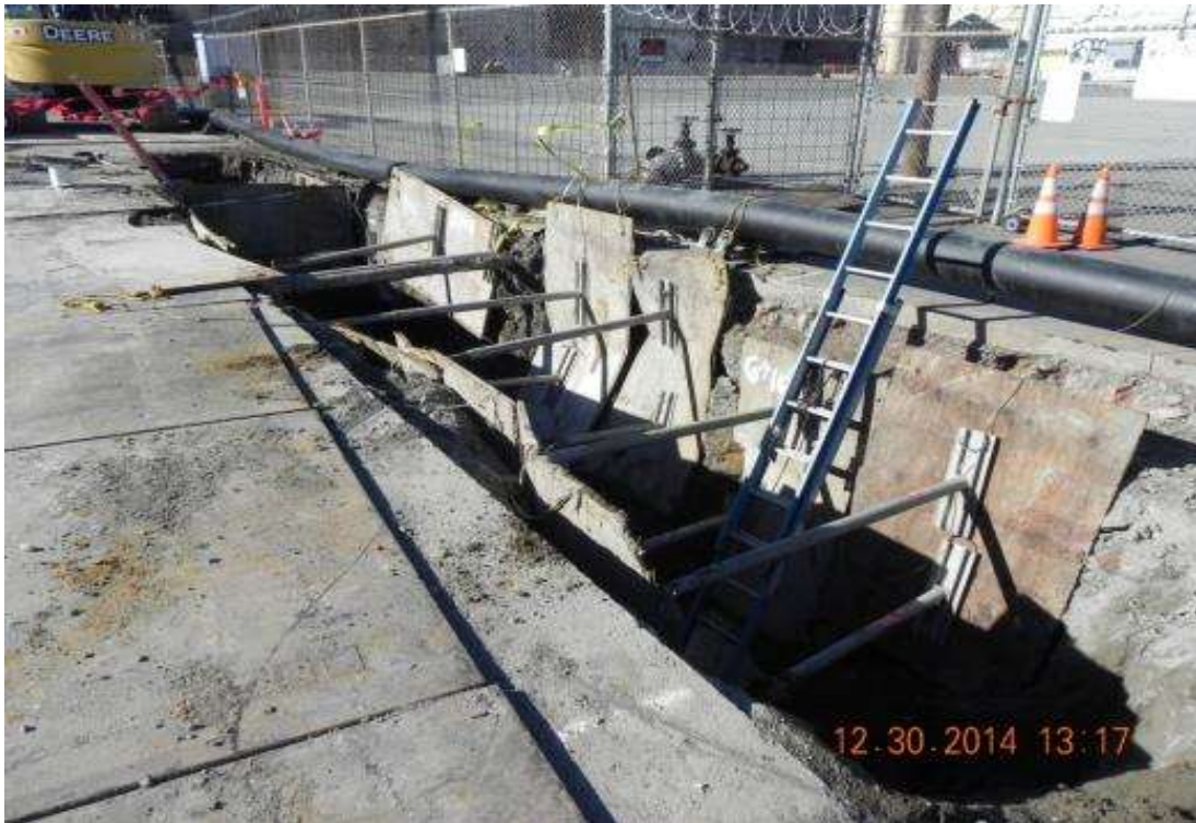
Figure 4 – Excavation and shoring for duct bank south on 23 rd Street. December 30, 2014. Photo courtesy of PG&E.
