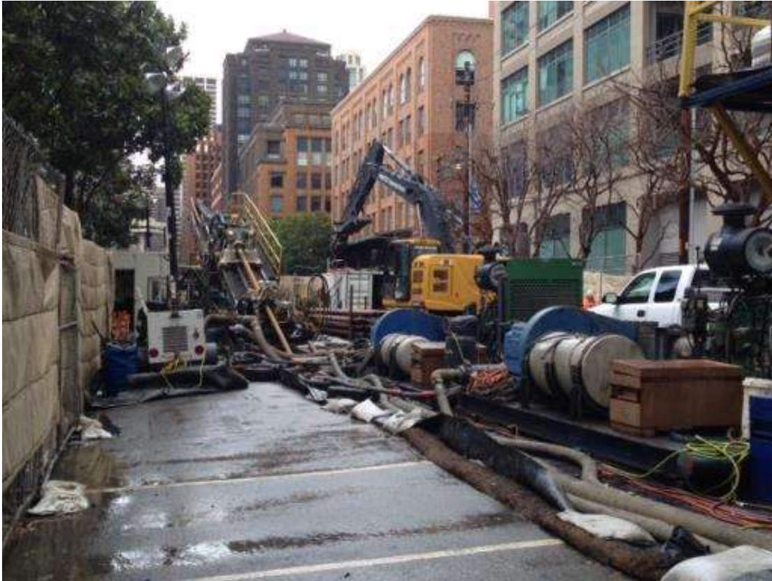
Figure 1 – HDD North equipment at Bore 1, view west, February 8, 2015. Photo courtesy of PG&E
