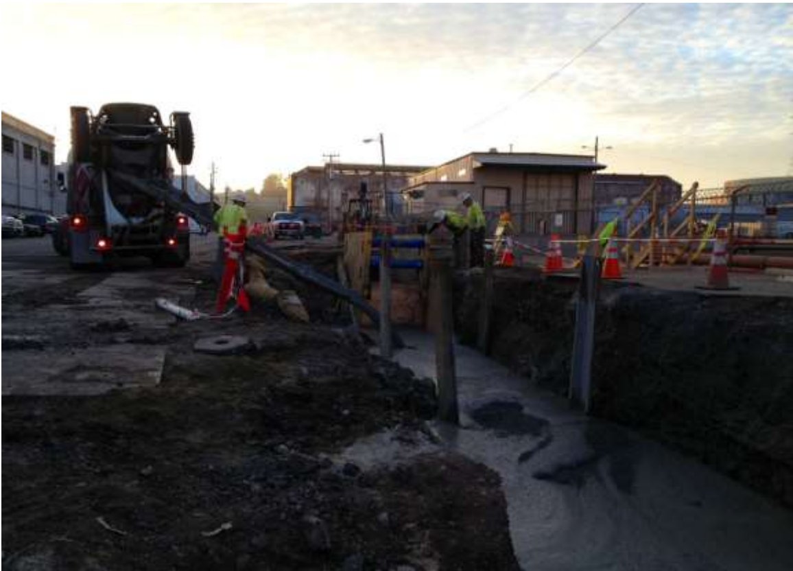
Figure 3 – Pouring cement slurry at underground duct bank on 23 rd Street. View west, February 2, 2015.
