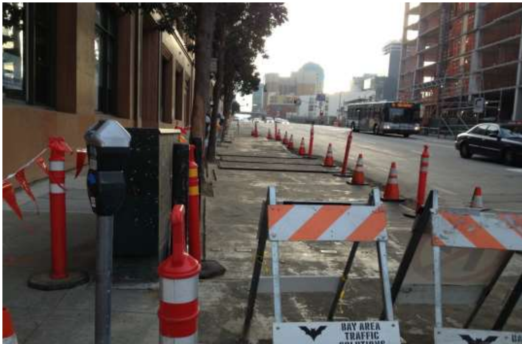
Figure 2 – Underground North duct bank on Folsom Street buttoned-up for the day. View south, February 2, 2015.
