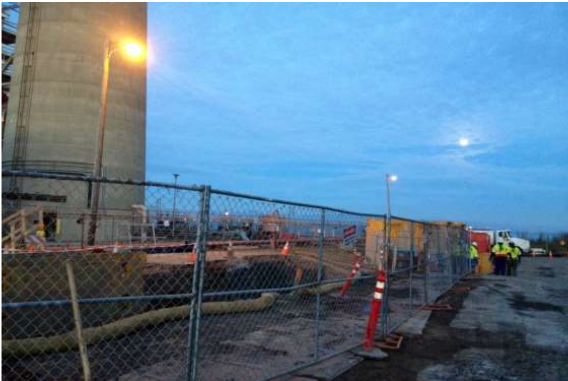
Figure 4 – Fencing installed at end of day around underground duct bank on 23 rd Street. View west, February 2, 2015.
