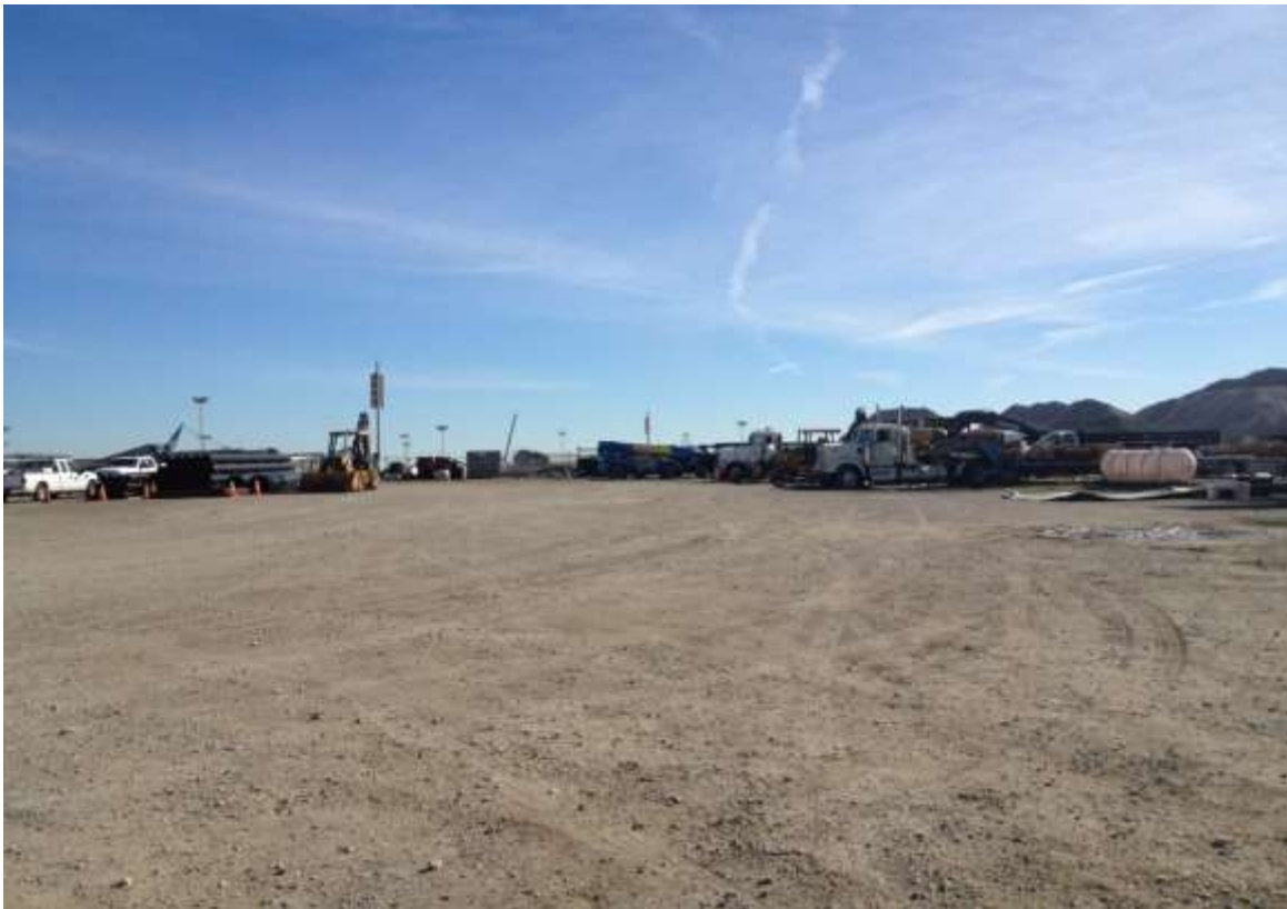
Figure 4 – Staging of equipment and materials at the Amador Yard. View south, February 12, 2015.
