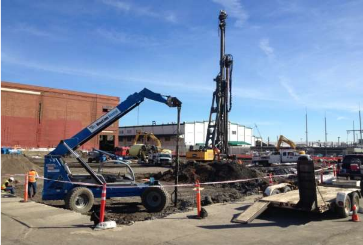
Figure 1 – Potrero Switchyard, view southeast, February 12, 2015.
