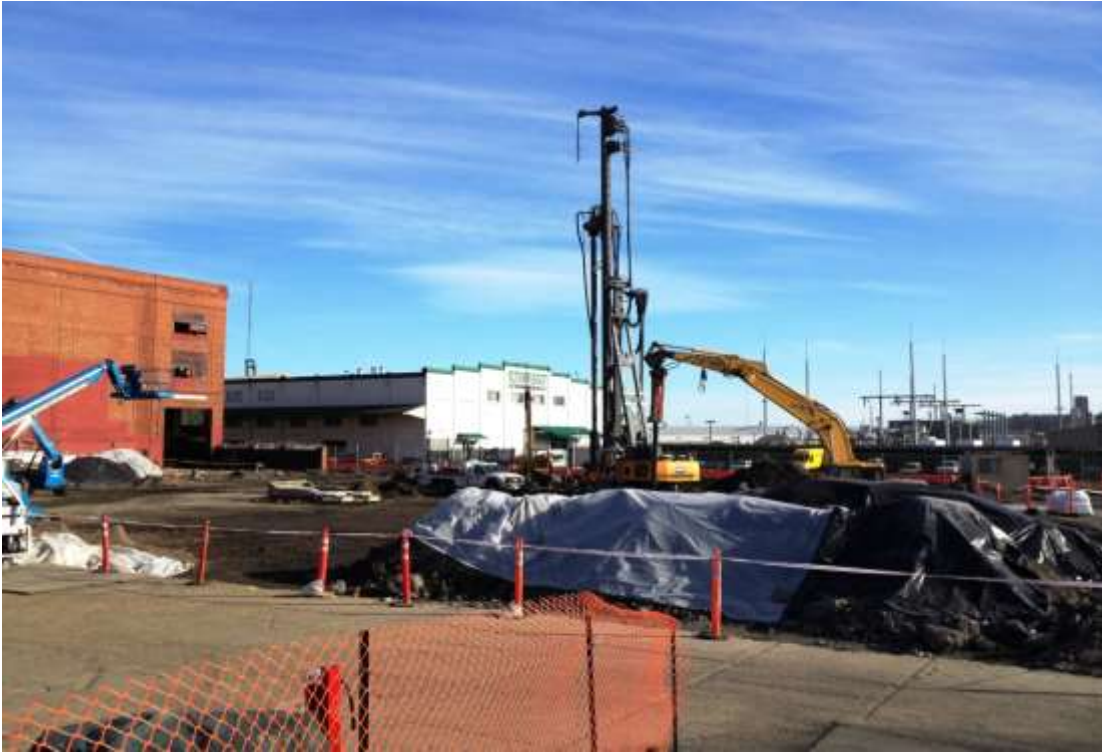
Figure 1 – Potrero Switchyard, view southeast, February 26, 2015.
