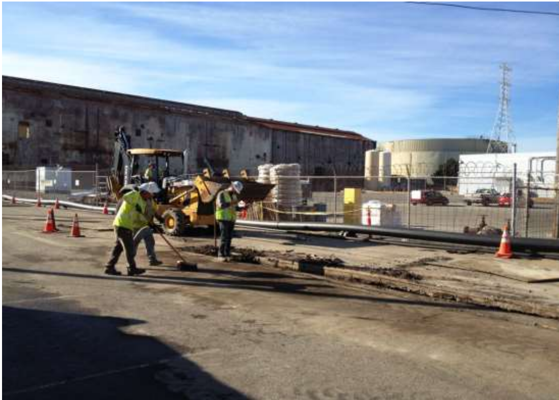
Figure 4 – Water line relocation work at Duct Bank South on 23 rd Street. View northwest, February 26, 2015.
