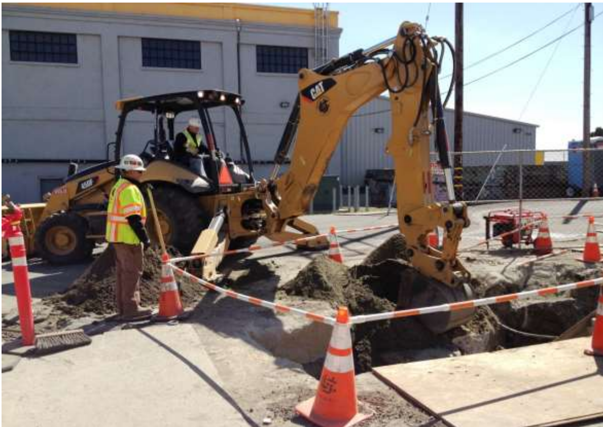
Figure 6 – Filling underground water circulation feature with sand on 23 rd Street. View southwest, April 1, 2015.
