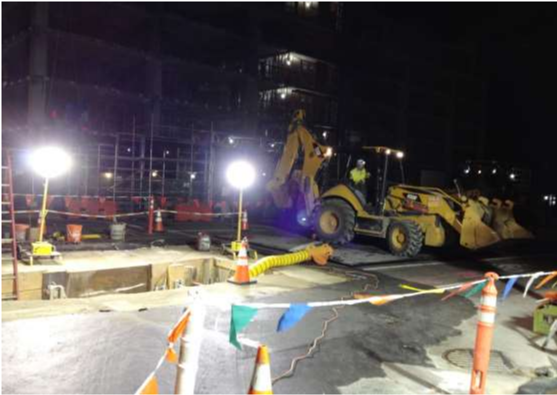
Figure 3 – Night work on underground duct bank at Folsom Street and Fremont Street. View northwest, April 1, 2015.
