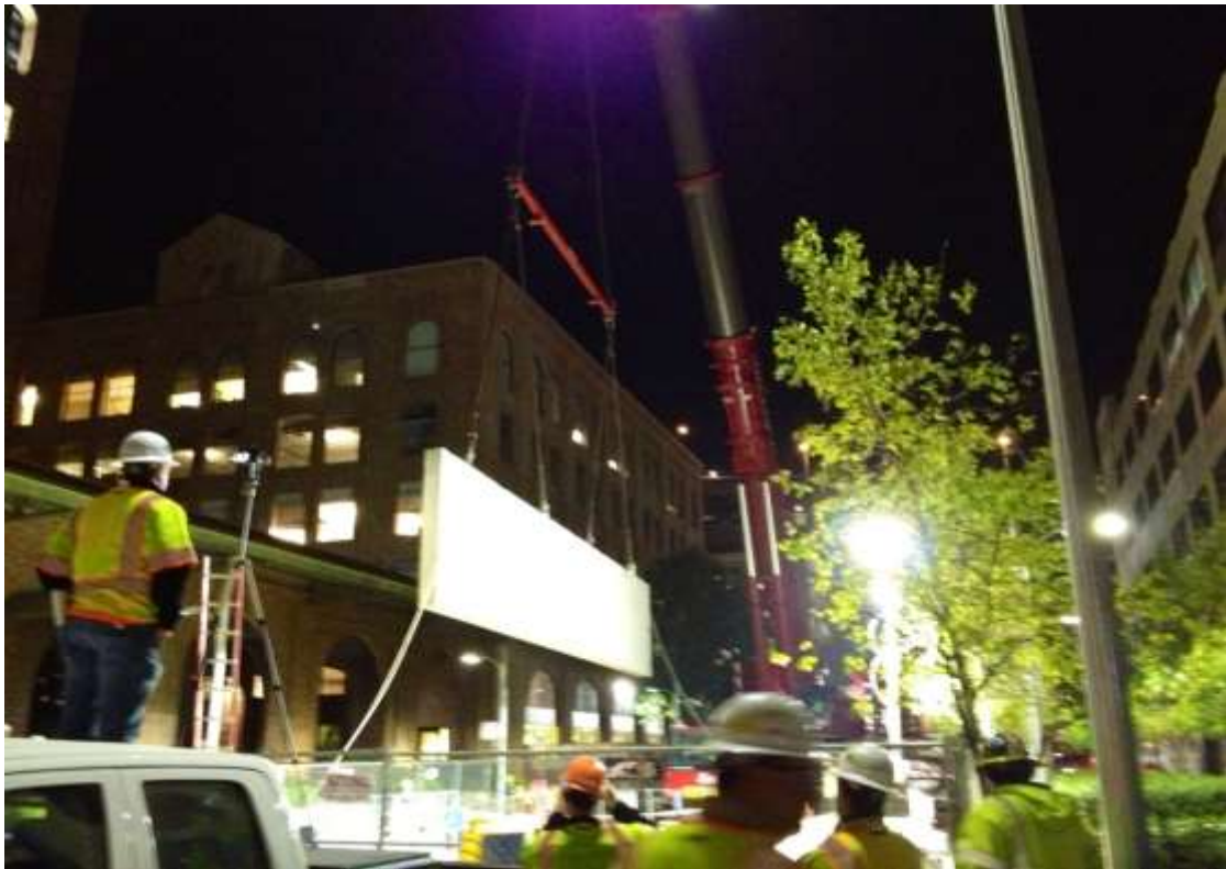
Figure 4 – Setting wall in vault with large crane on Spear Street. View east, April 1, 2015.
