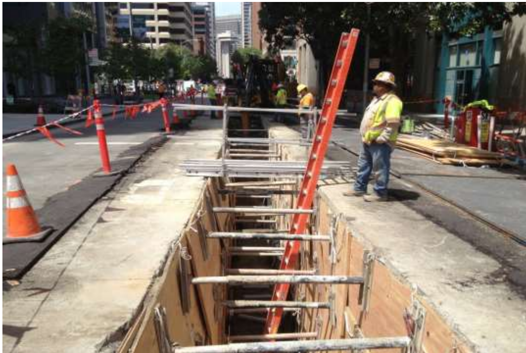
Figure 2 – Excavating duct bank trench on Spear Street west of vault. View west, April 28, 2015.
