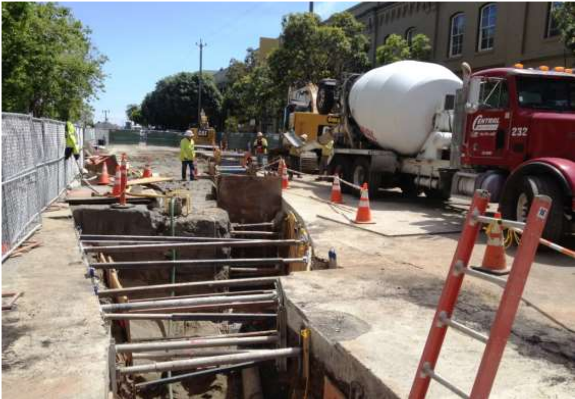
Figure 3 – Pouring cement slurry in duct bank trench at HDPE transition on Spear St. View east, April 28, 2015.
