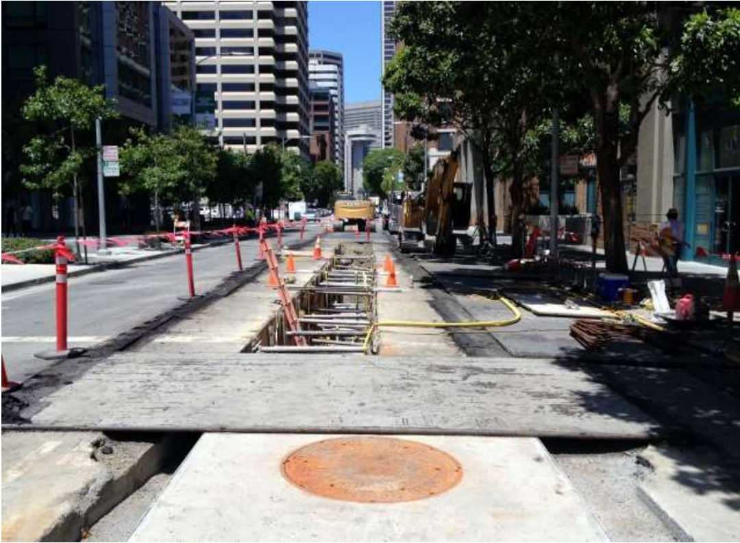
Figure 1 – Excavating duct bank trench on Spear Street between vault and Folsom Street. View west, June 4, 2015.
