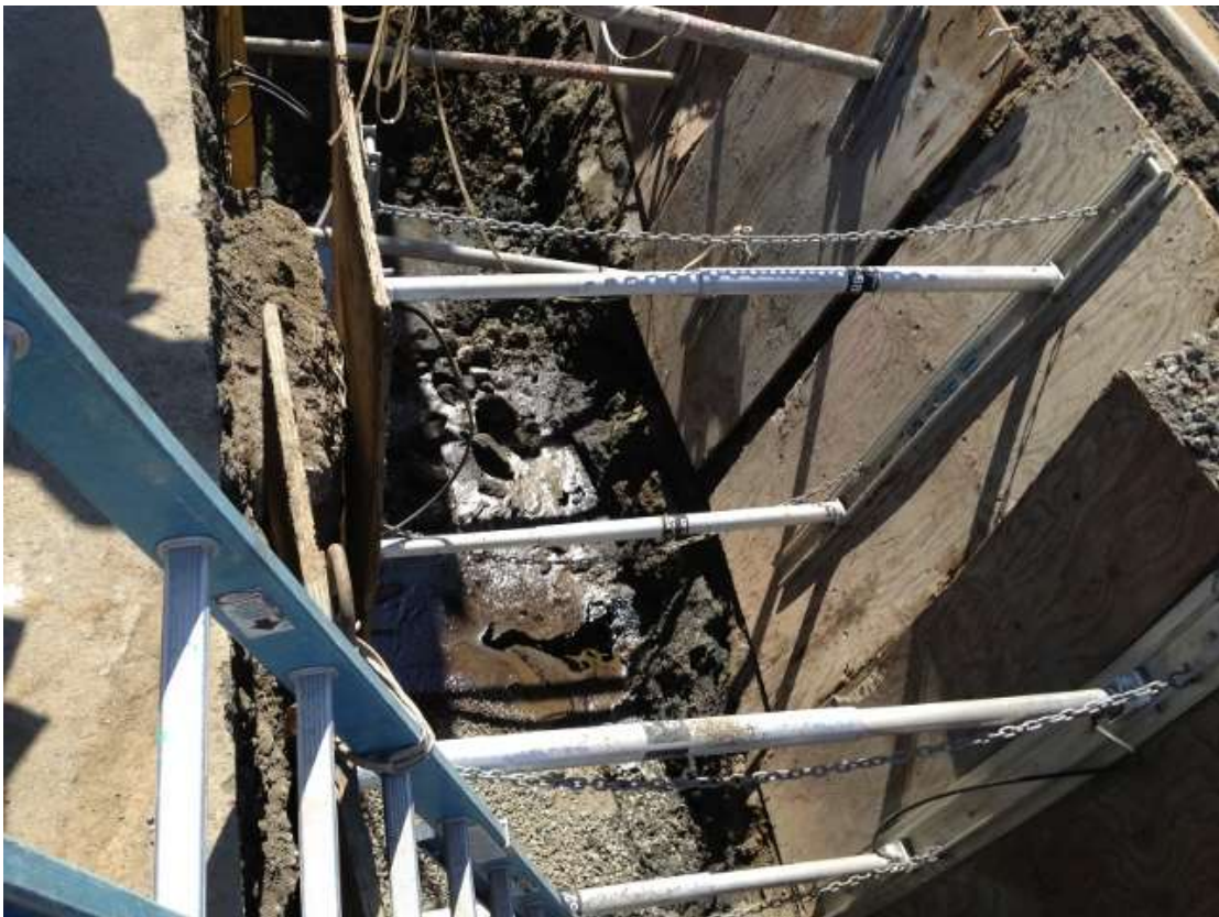
Figure 4 – Oily black substance in trench on 23 rd Street. View northwest, June 4, 2015.
