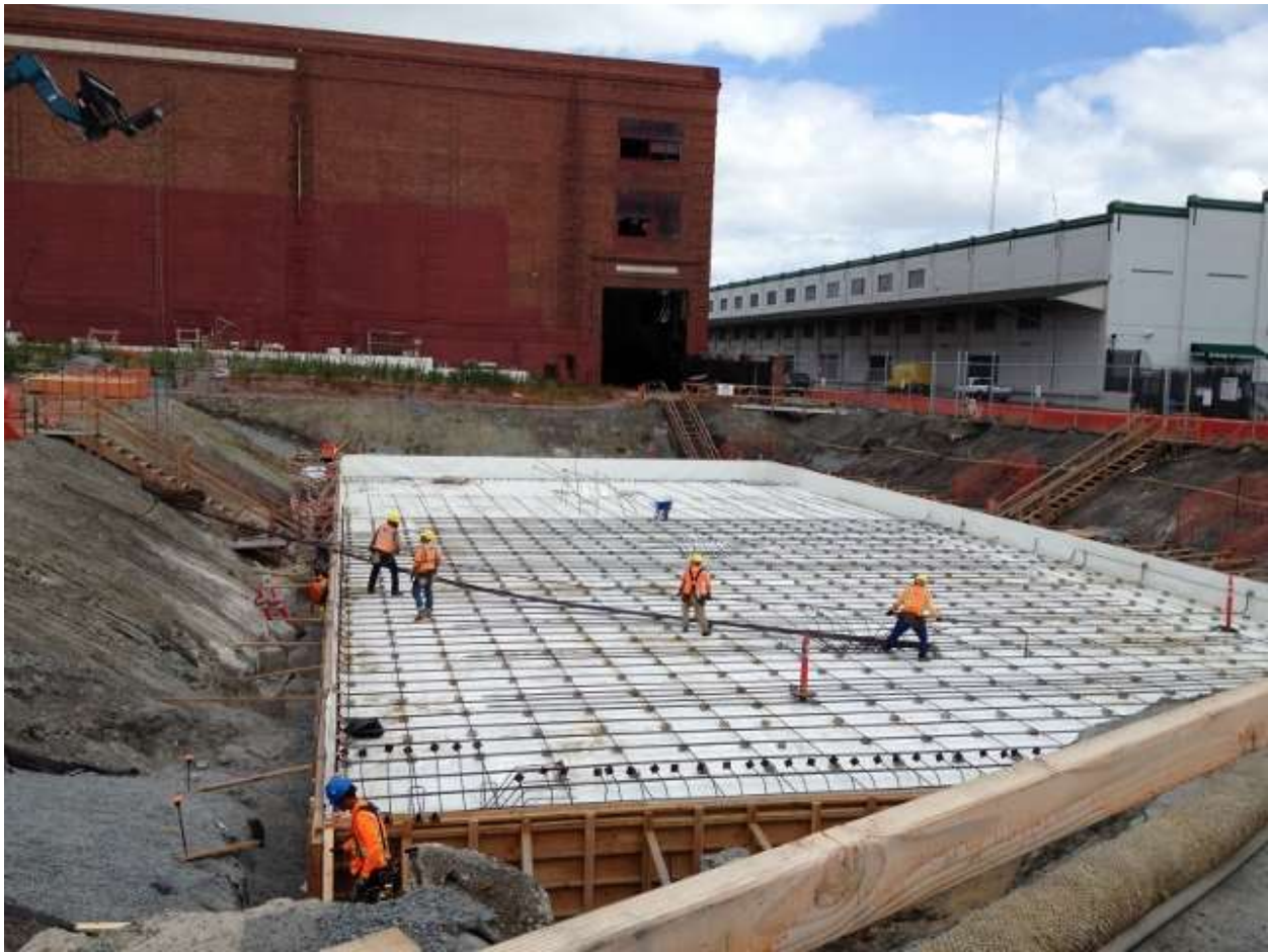
Figure 3 – Crews laying out rebar for GIS building foundation at Potrero Switchyard. View southeast, July 10, 2015.
