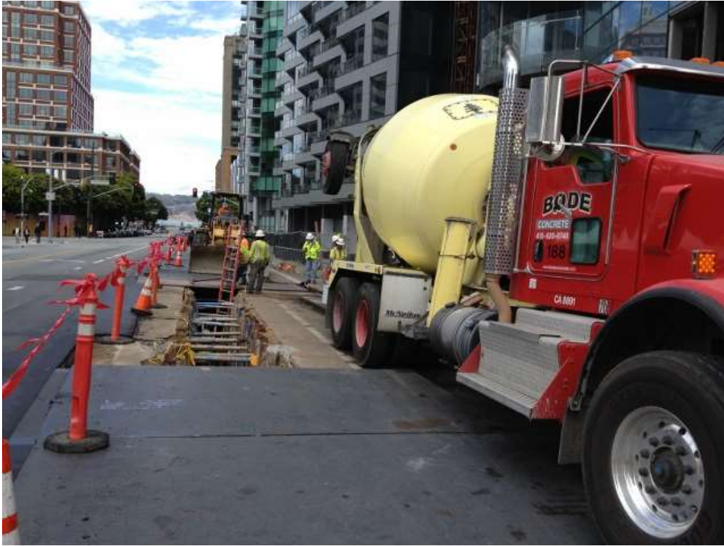
Figure 1 – Duct Bank North work on Folsom Street between Beale Street and Main Street. View north, July 10, 2015.
