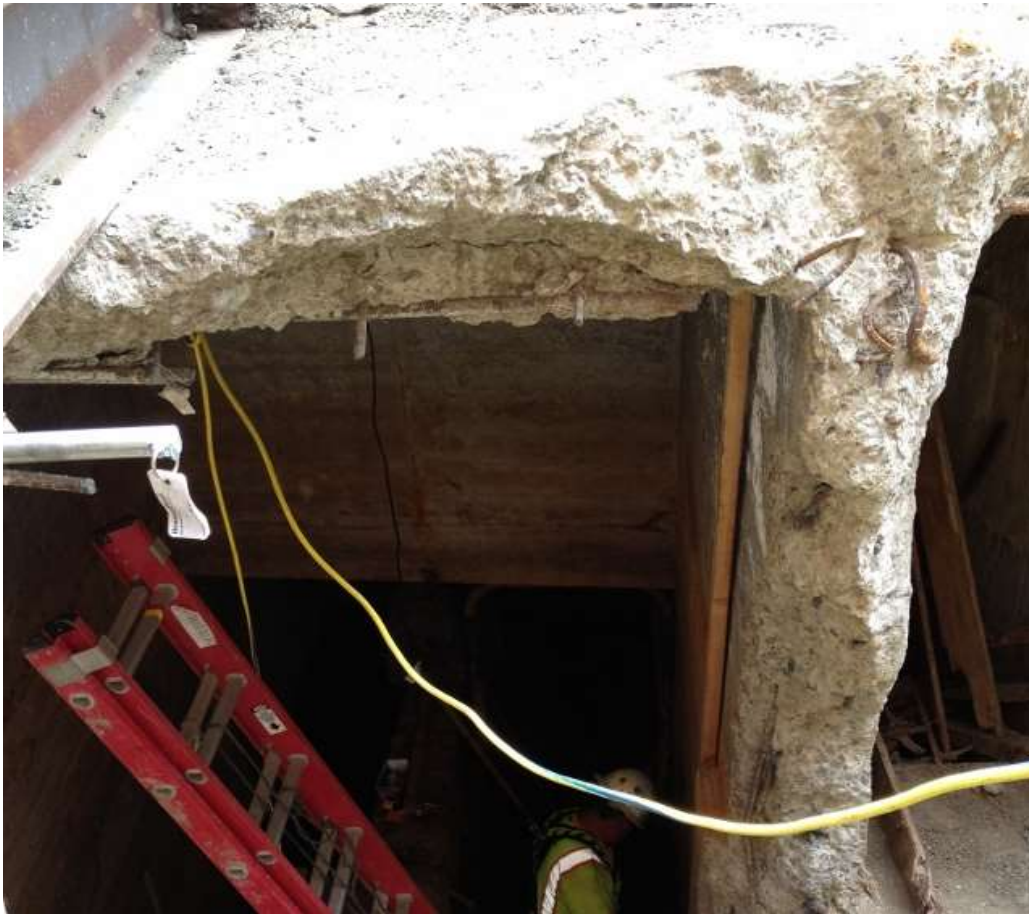
Figure 4 – Building wall in Station A water circulation vault feature for duct bank trench on 23 rd Street. View south, August 21, 2015.
