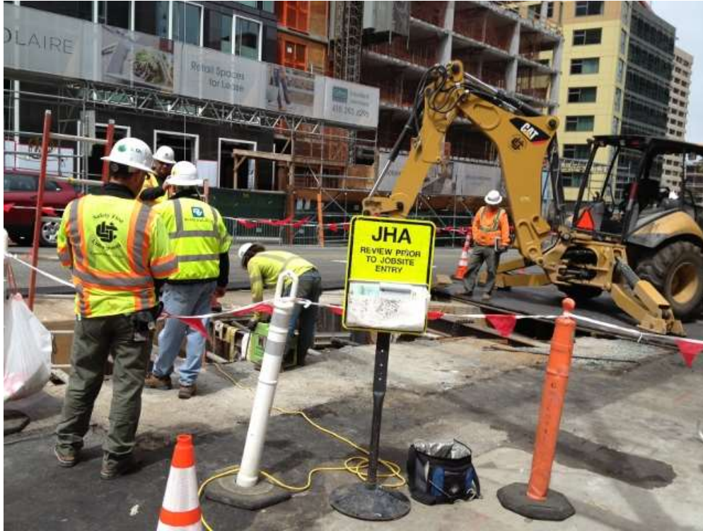
Figure 1 – Excavating and shoring the duct bank trench on Folsom Street near Fremont Street. View northwest, August 21, 2015.
