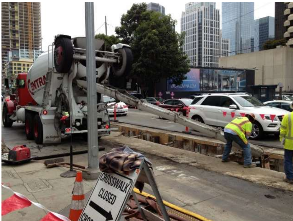
Figure 2 – Backfilling trench with cement slurry on Folsom Street near Spear Street. View southwest, August 21, 2015.
