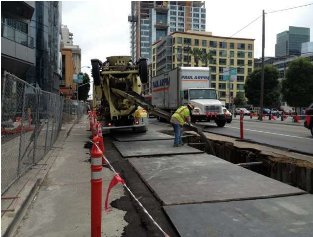
Figure 3 – Pouring concrete on Folsom Street between Beale and Main Streets. View south, September 14, 2015.
