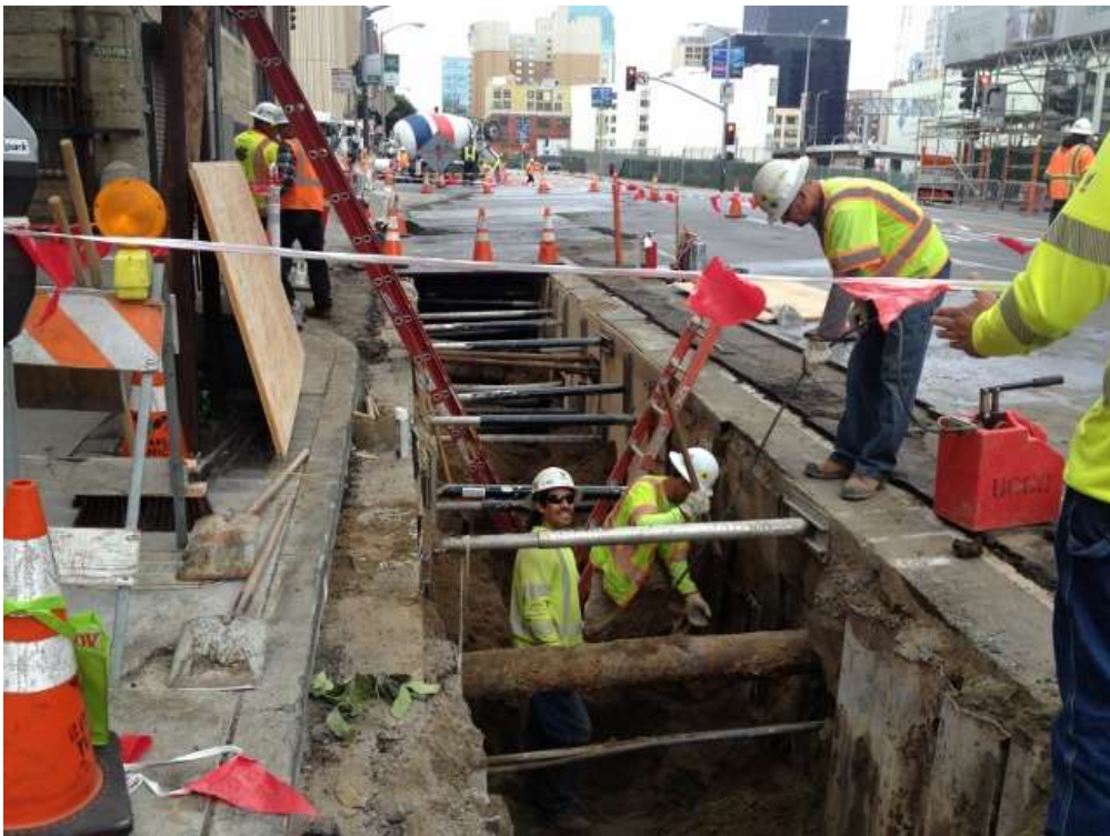
Figure 2 – Excavating on Folsom Street between Fremont and Beale Streets. View south, September 14, 2015.
