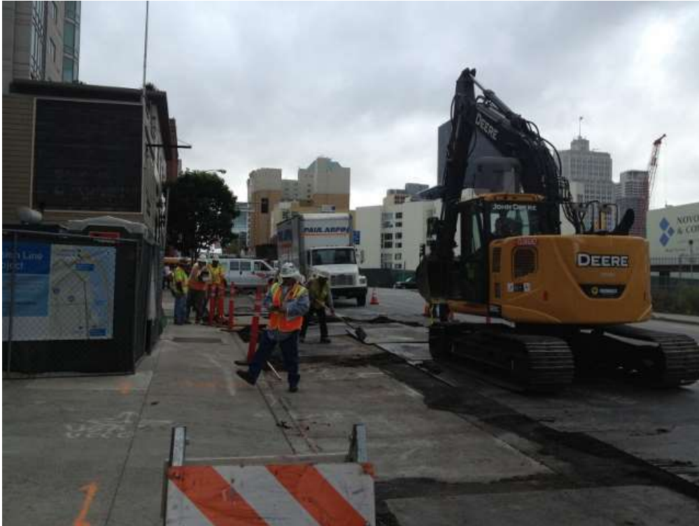
Figure 1 – Excavating duct bank trench on Folsom Street between 1 st Street and Fremont Street. View south, September 14, 2015.
