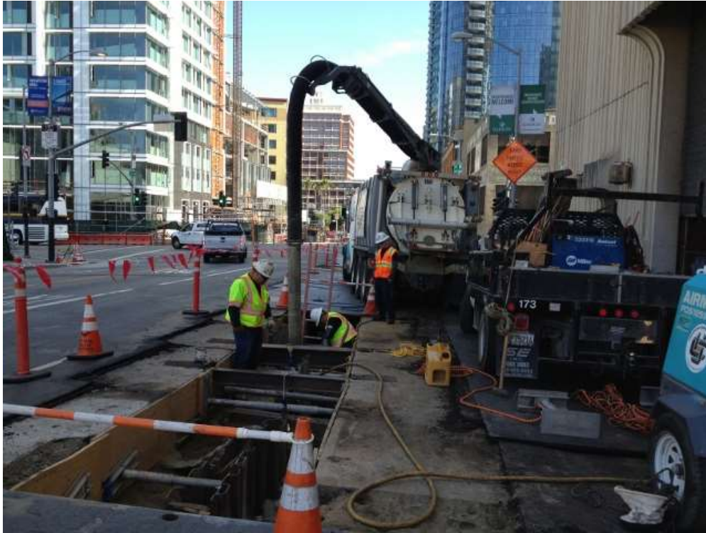
Figure 1 – Excavating the duct bank trench with a Vac-truck on Folsom Street just south of Fremont Street. View North, October 6, 2015.
