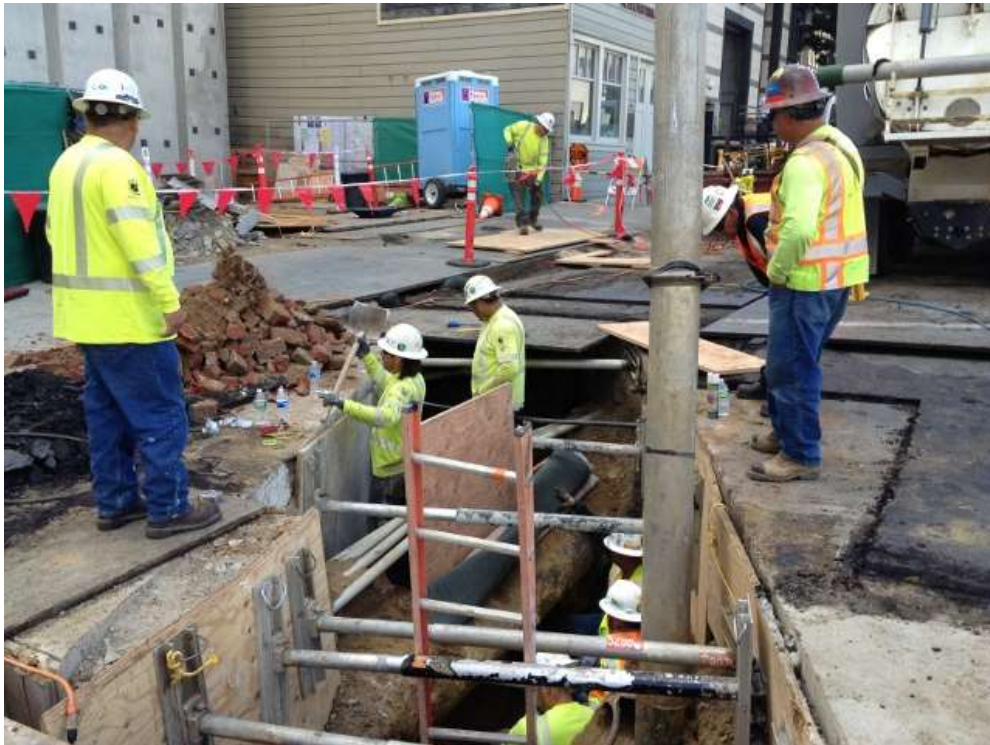
Figure 2 – Exposing 16-inch gas pipeline just outside the Embarcadero Substation. View southeast, October 6, 2015.
