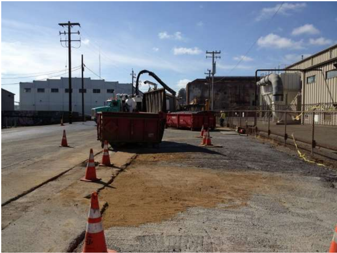
Figure 5 – Dried spoils spill from roll off bin on 23 rd Street. View north, October 6, 2015.
