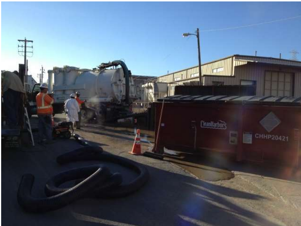
Figure 4 – PSC working on cleaning up spoils spill on 23 rd Street. View west, November 3, 2015.
