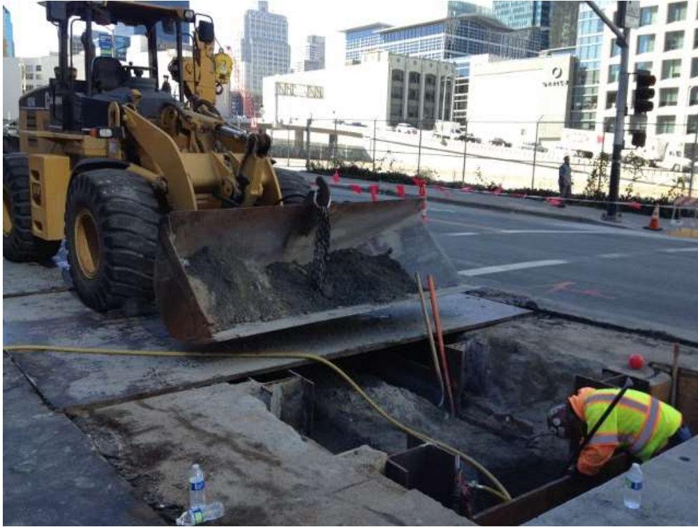
Figure 1 – Exposing I-beam shoring on Folsom Street in front of Embarcadero Substation. View southwest, November 3, 2015.
