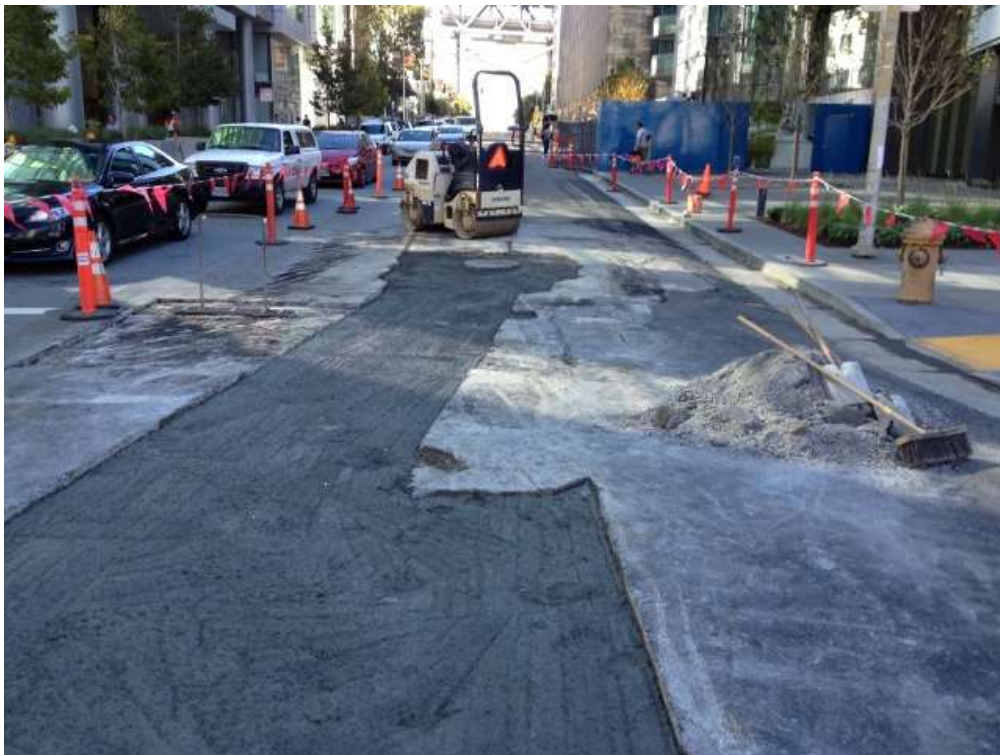
Figure 2 – Backfilling with cement at Main and Folsom Streets intersection. View east, November 3, 2015.
