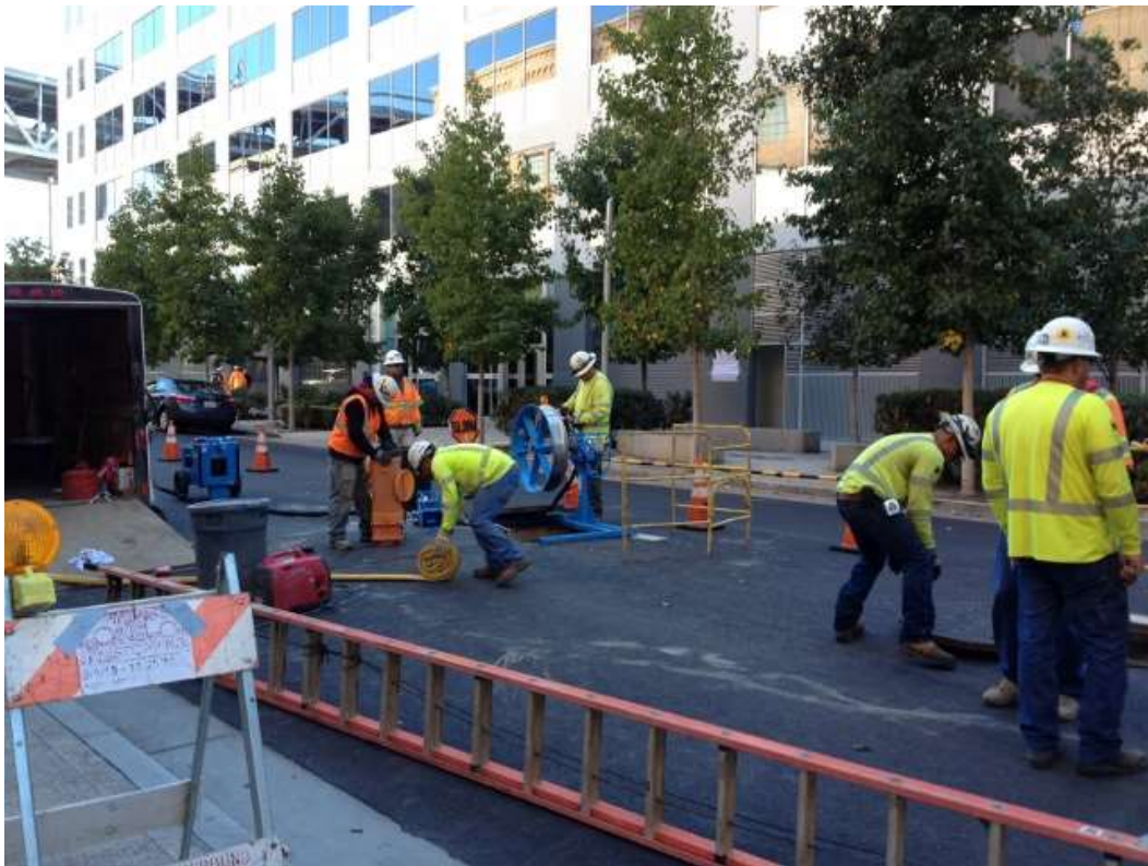
Figure 3 – Installing mule tape and mandreling conduit at transition vault on Spear Street. View southeast, November 3, 2015.
