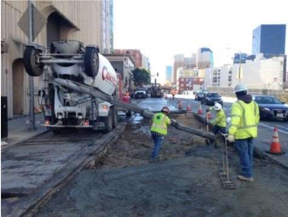
Figure 1 – Backfilling trench with concrete on Folsom Street in front of Embarcadero Substation. View southwest, November 10, 2015. Photo courtesy of PG&E.
