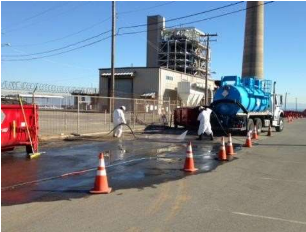
Figure 3 – PSC cleaning up spill from roll-off bins on 23 rd Street. View east, November 13, 2015. Photo courtesy of PG&E.
