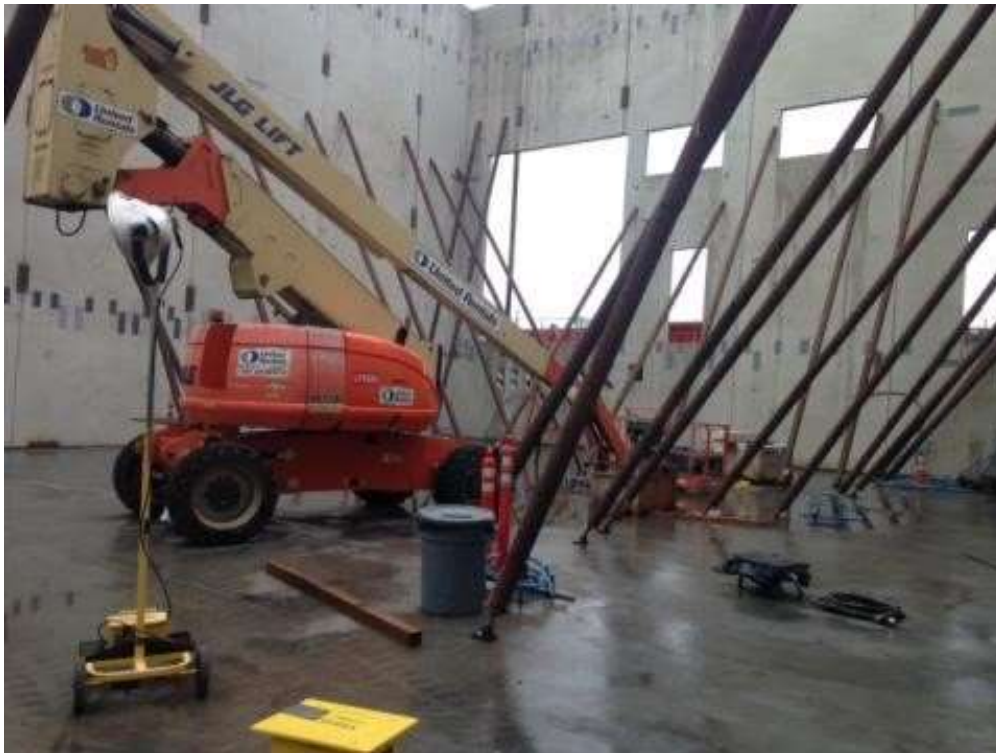
Figure 4 – Inside GIS Building at the Potrero Switchyard. View northeast, November 9, 2015. Photo courtesy of PG&E.
