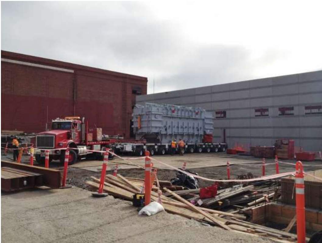
Figure 3 – Transformer being staged next to GIS building Potrero Switchyard. View southeast, December 17, 2015.
