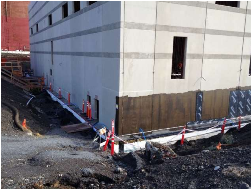
Figure 4 – Stormwater draining well around GIS building in Switchyard. View southeast, January 7, 2016.
