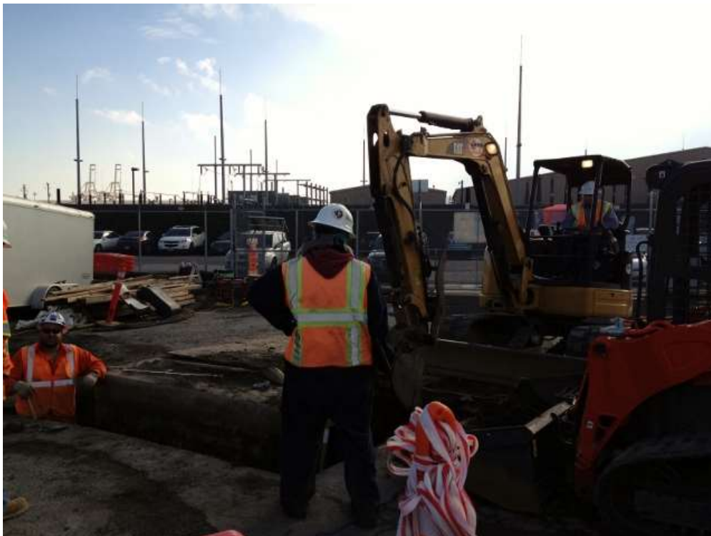
Figure 2 – Crew excavating around old foundation for removal within Switchyard. View south, January 7, 2016.
