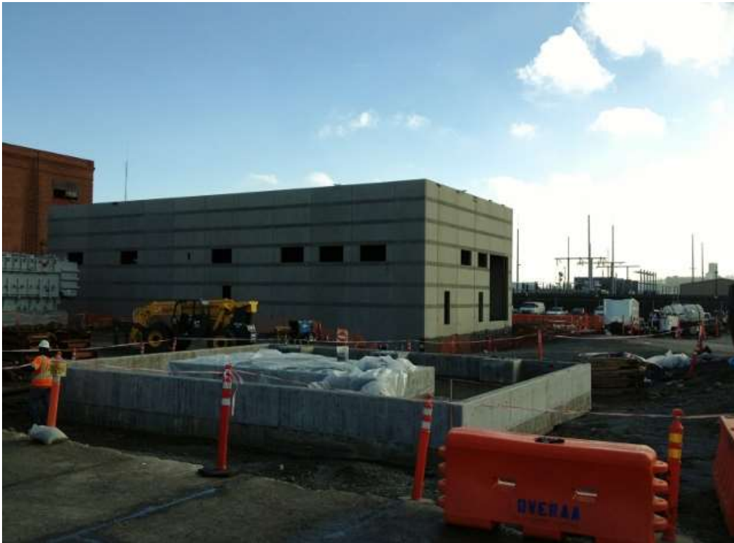
Figure 3 – Crews working on removing forms from reactor pad in Switchyard. View southeast, January 7, 2016.
