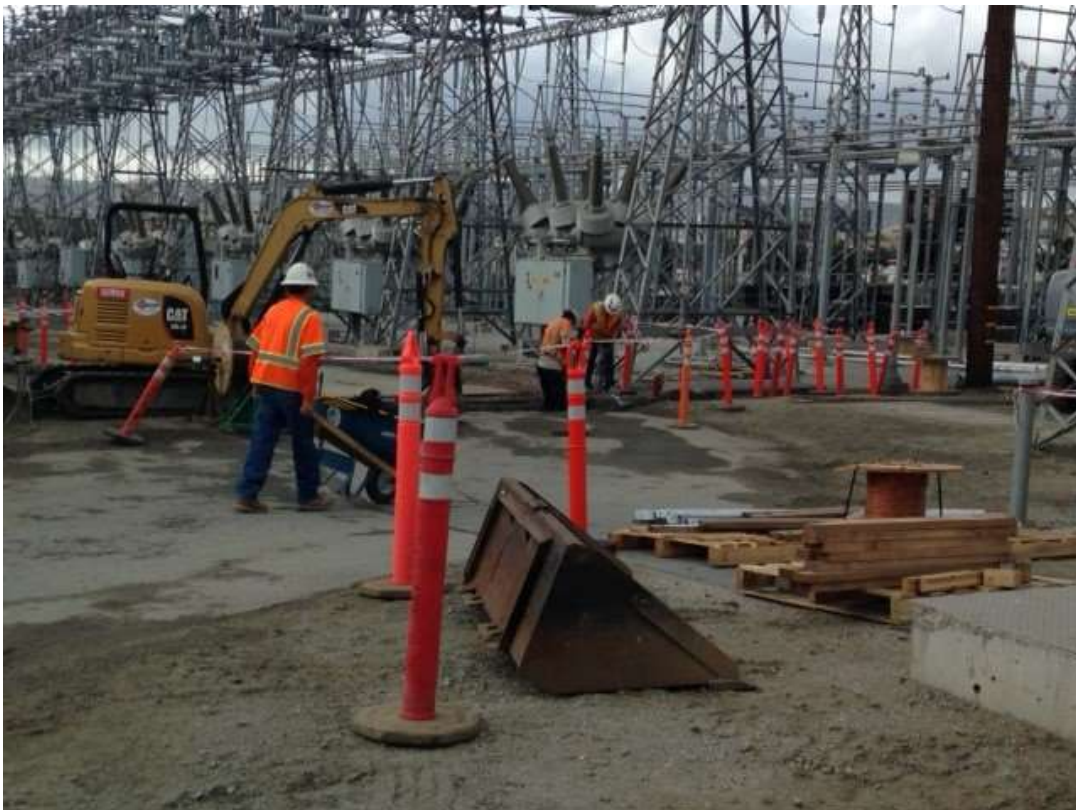
Figure 4 – APEC excavated in the substation. View southwest, February 17, 2016. Photo courtesy of PG&E.
