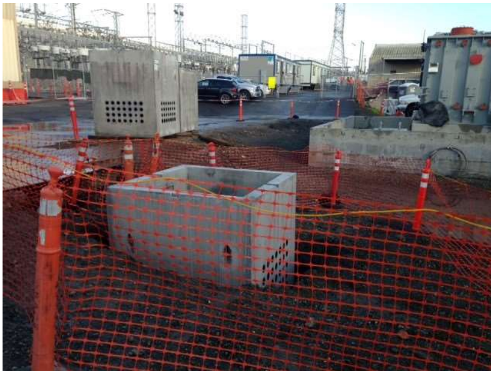
Figure 2 – APEC installed an electrical box in the cable trench. View north, February 18, 2016. Photo courtesy of PG&E.
