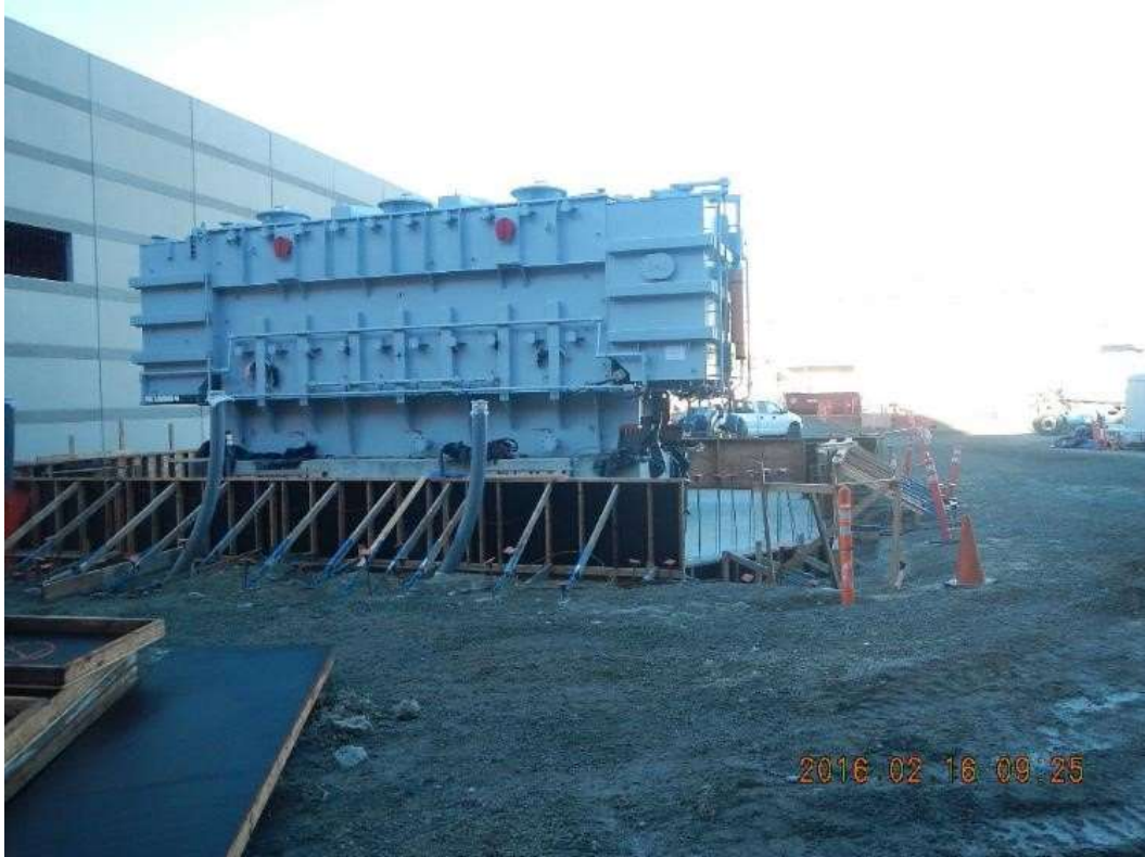
Figure 3 – APEC installed forms and/or rebar at the transformer pad. View west, February 16, 2016. Photo courtesy of PG&E.
