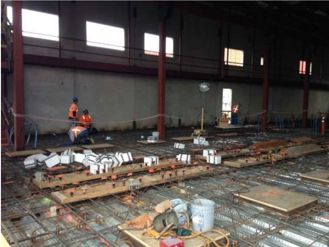
Figure 1 – Metal Set welded in the GIS building. View northeast, February 17, 2016. Photo courtesy of PG&E.
