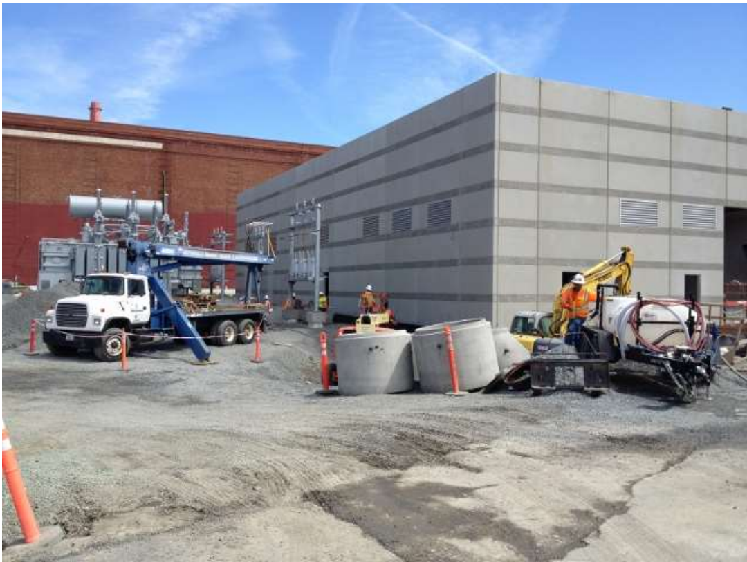
Figure 3 – Crews installed metal infrastructure north of the GIS building. View southeast, April 20, 2016.
