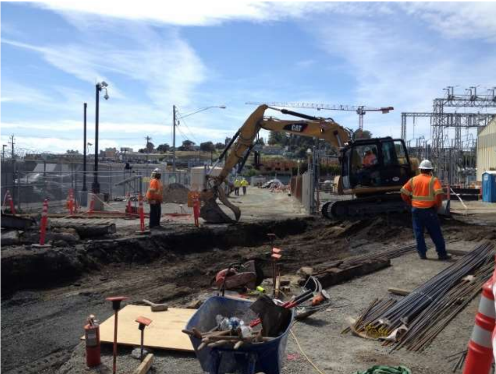
Figure 2 – Crews excavated trench for cable installation between the GIS building and the substation. View west, April 20, 2016.
