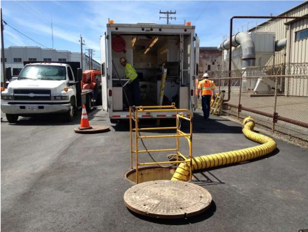
Figure 1 – Crews racking in the transition vault of 23 rd Street. View west, April 20, 2016.
