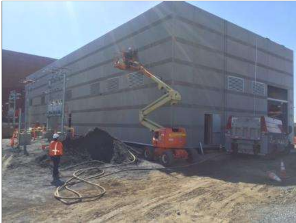
Figure 1: MEI installing light fixtures on the GIS building in the Potrero Switchyard, May 16, 2016. Photo courtesy of PG&E.
