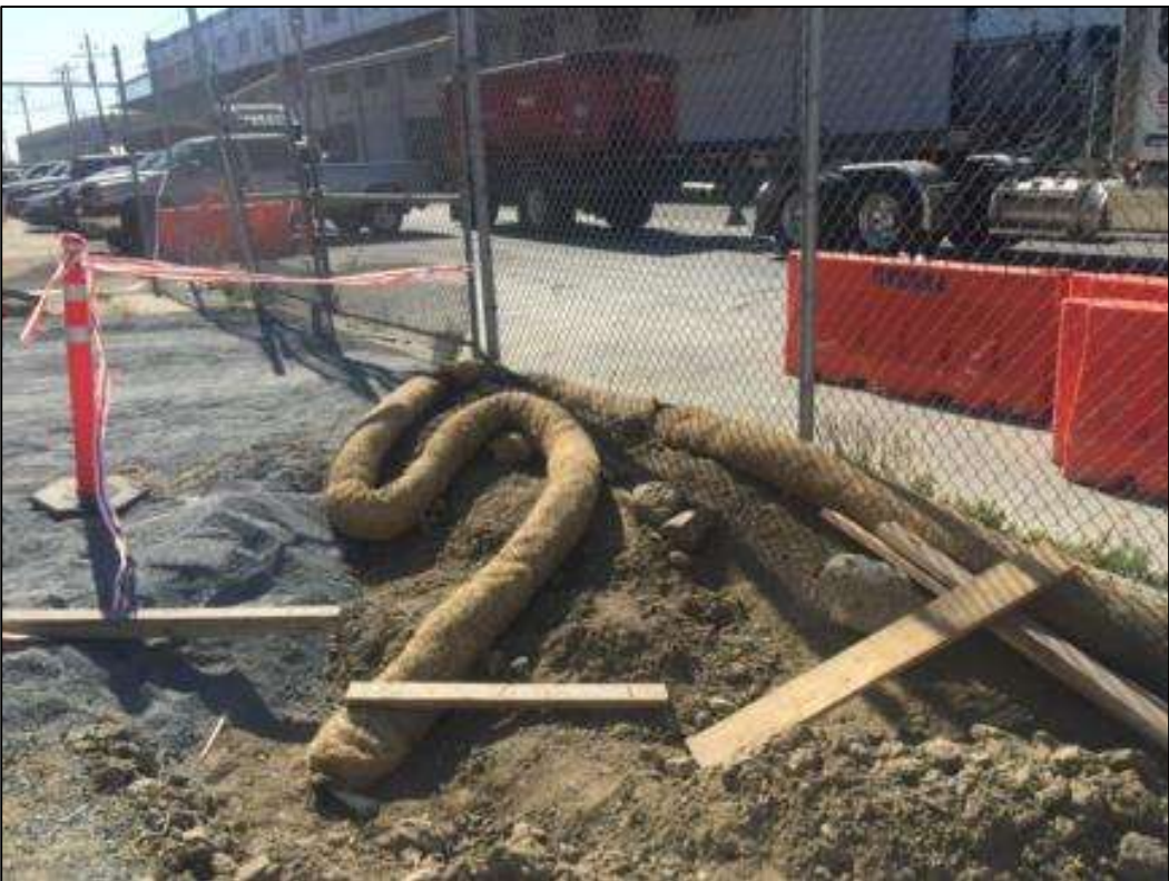
Figure 4: Fiber roll installed on top of dirt at curb at eastern 23rd St. gate at Potrero Switchyard, May 16, 2016. Photo courtesy of PG&E.
