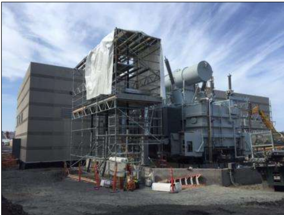
Figure 2: Scaffolding Solutions installing plastic around scaffolding at the transformer in the Potrero Switchyard, May 19, 2016. Photo courtesy of PG&E.
