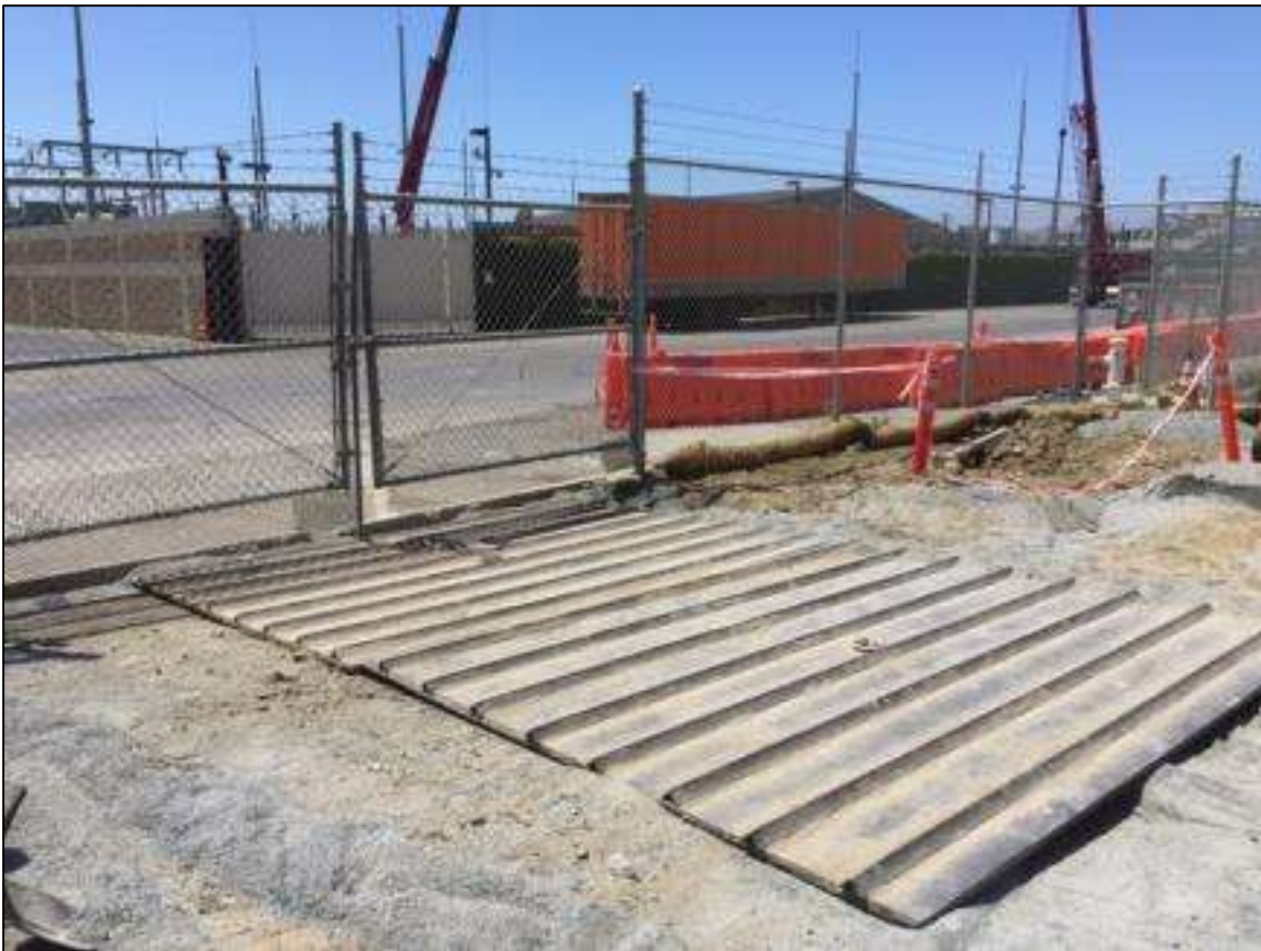
Figure 5: Rumble plate installed at new 23rd St gate in the Potrero Switchyard, May 18, 2016. Photo courtesy of PG&E.
