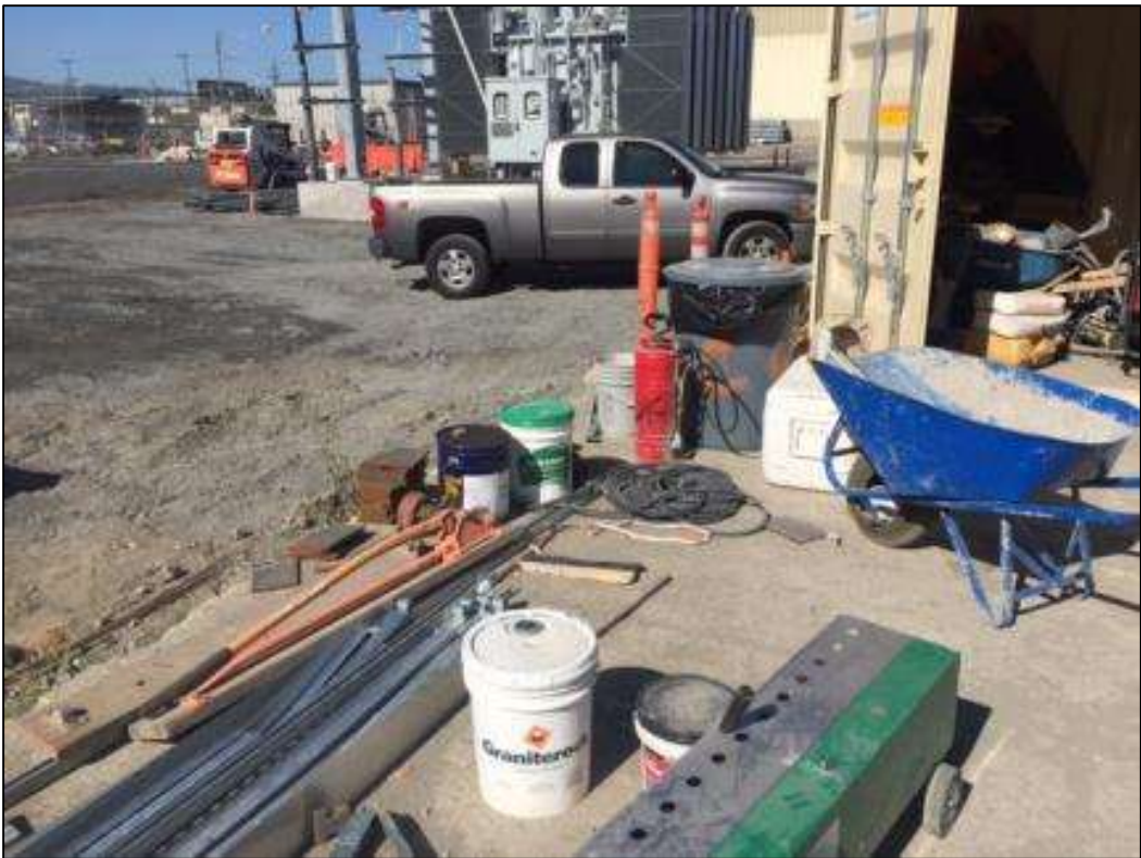
Figure 3: Hazardous materials without containment in the Potrero Switchyard, May 17, 2016. Photo courtesy of PG&E.
