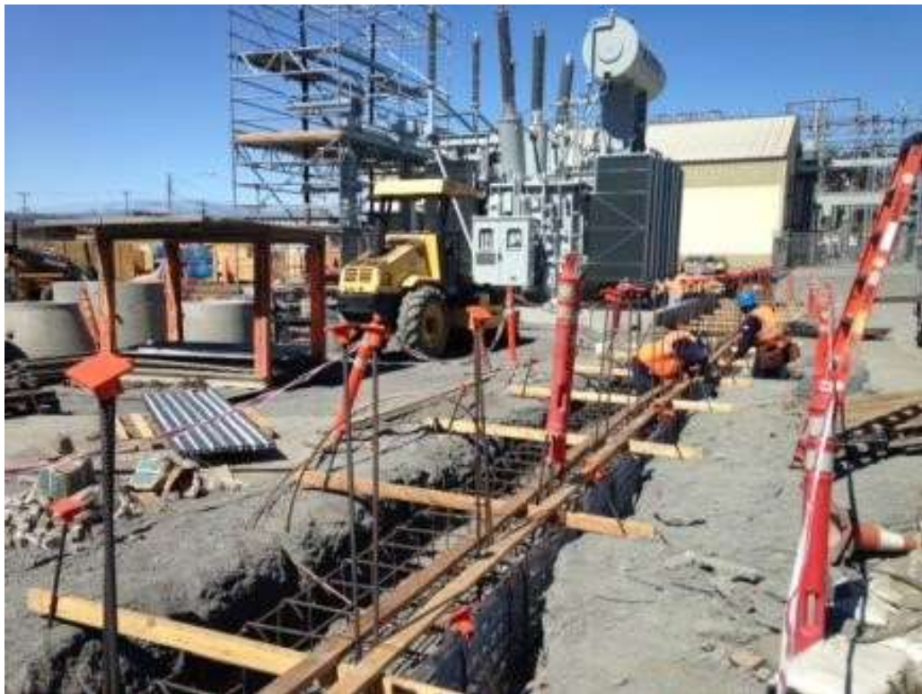
Figure 2: Overaa installing rebar in the perimeter wall excavation, June 27, 2016. Photo courtesy of PG&E.
