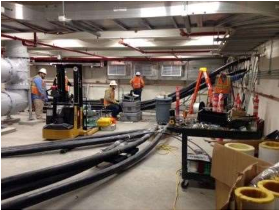
Figure 3: PG&E camera scoped conduit in the GIS building basement, June 27, 2016. Photo courtesy of PG&E.
