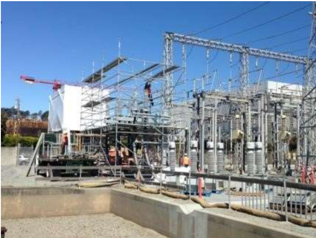
Figure 4: SSI removed scaffolding around the 115 kV bus in the substation, June 27, 2016. Photo courtesy of PG&E.
