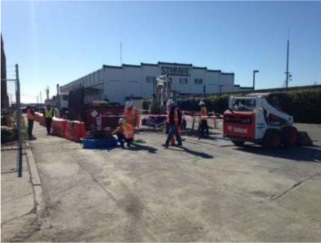
Figure 1: APEC excavating for the water and sewer line tie-in on 23 rd Street, June 27, 2016. Photo courtesy of PG&E.
